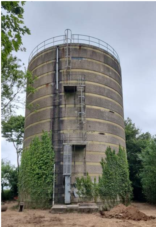
1.8 Tower Structural Images – minor spalling and clear signs of maintenance
