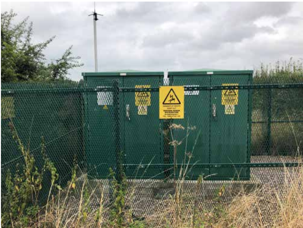
Electrical substation at north-western Site boundary
