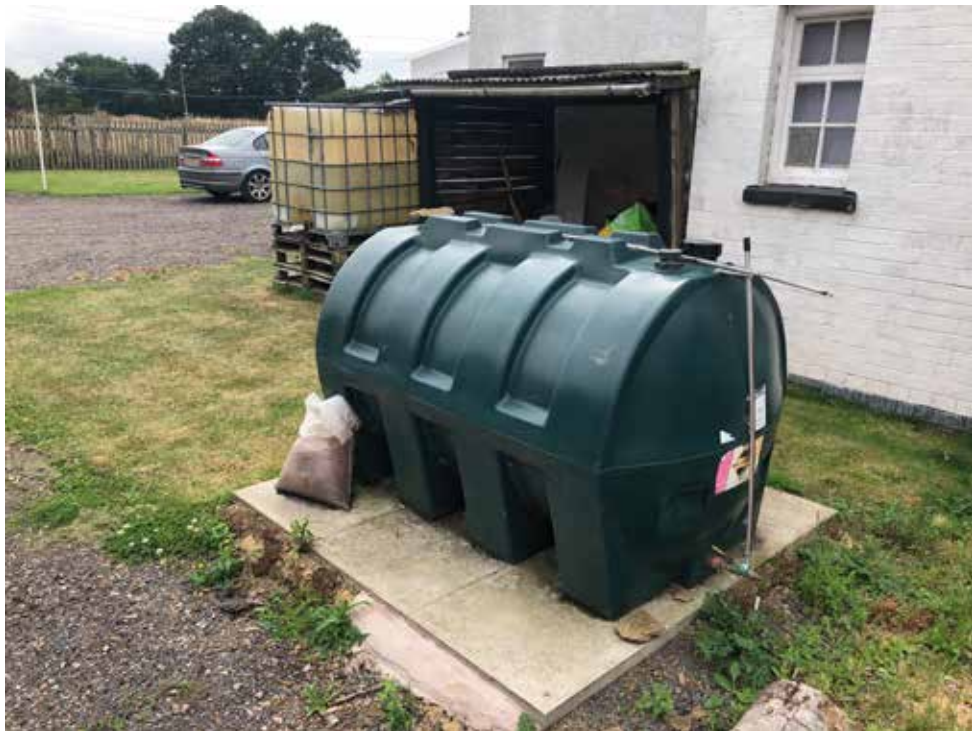
Oil storage tank at The Elms Farm
