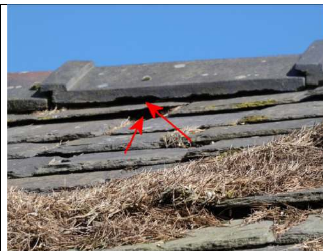
Photograph 35. Example of openings under ridge tiles and slates on the roof of the outbuilding
