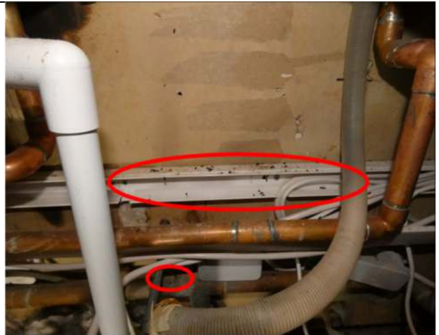
Photograph 20. Further example of bat droppings in the boiler room to the east of the westernmost north facing dormer window
