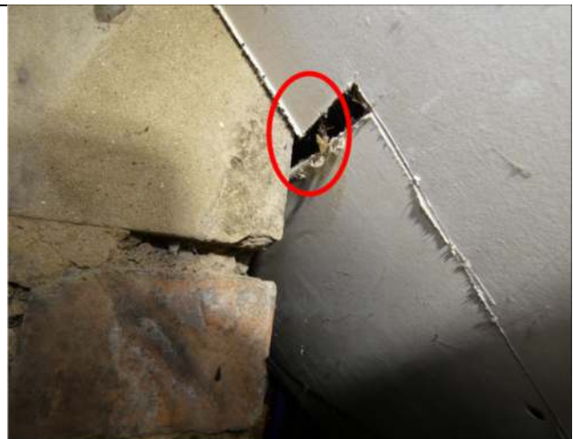
Photograph 28. Bat droppings caught in an opening within the western section of enclosed roof void under the chimney
