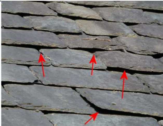
Photograph 9. Example of openings under slates on the roof of the single-storey extension at the south-west corner of the house
