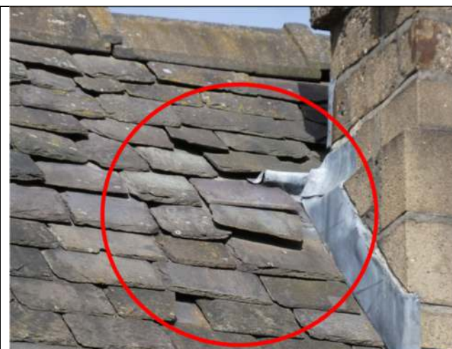
Photograph 29. Openings under slates near the base of the chimney
