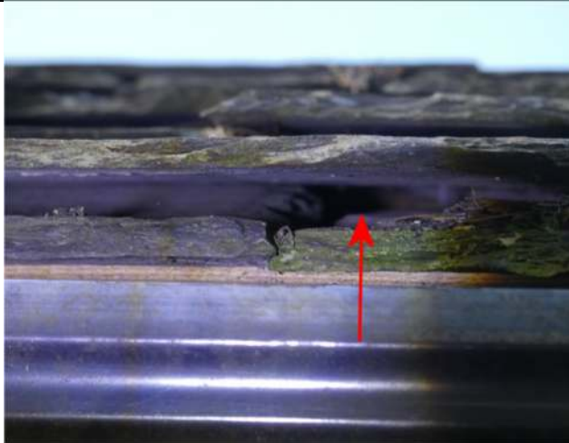
Photograph 37. Further example of an opening under a slate on the roof of the outbuilding
