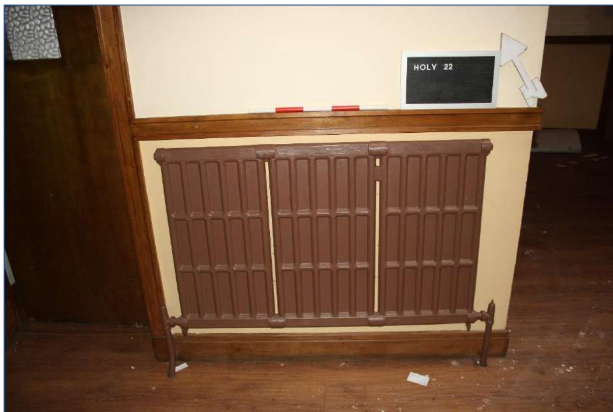
Plate 52: Radiator detail Room 5 looking E.
