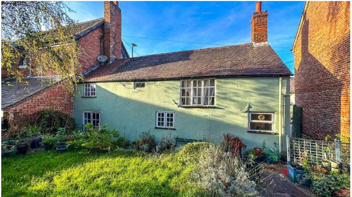
Rear view of cottage. All windows to be replaced due to rotting. French door proposal to replace middle window into utility room for access and natural light/ ventilation.
