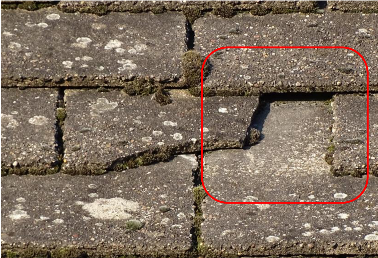
Image 2 – Further gaps of value to bats within the roof coverings above the garage section of the property, South facing elevation
