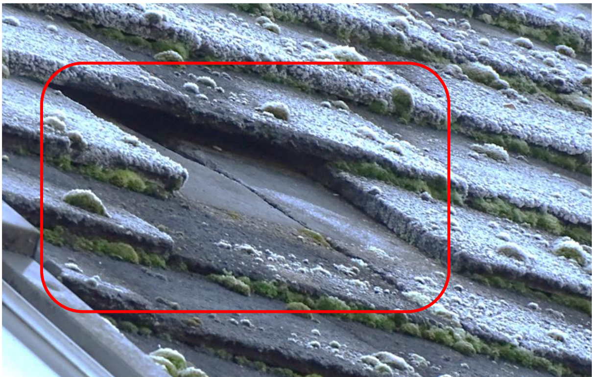
Image 6 – Further gaps of value to bats within the roof coverings to the rear North facing elevation
