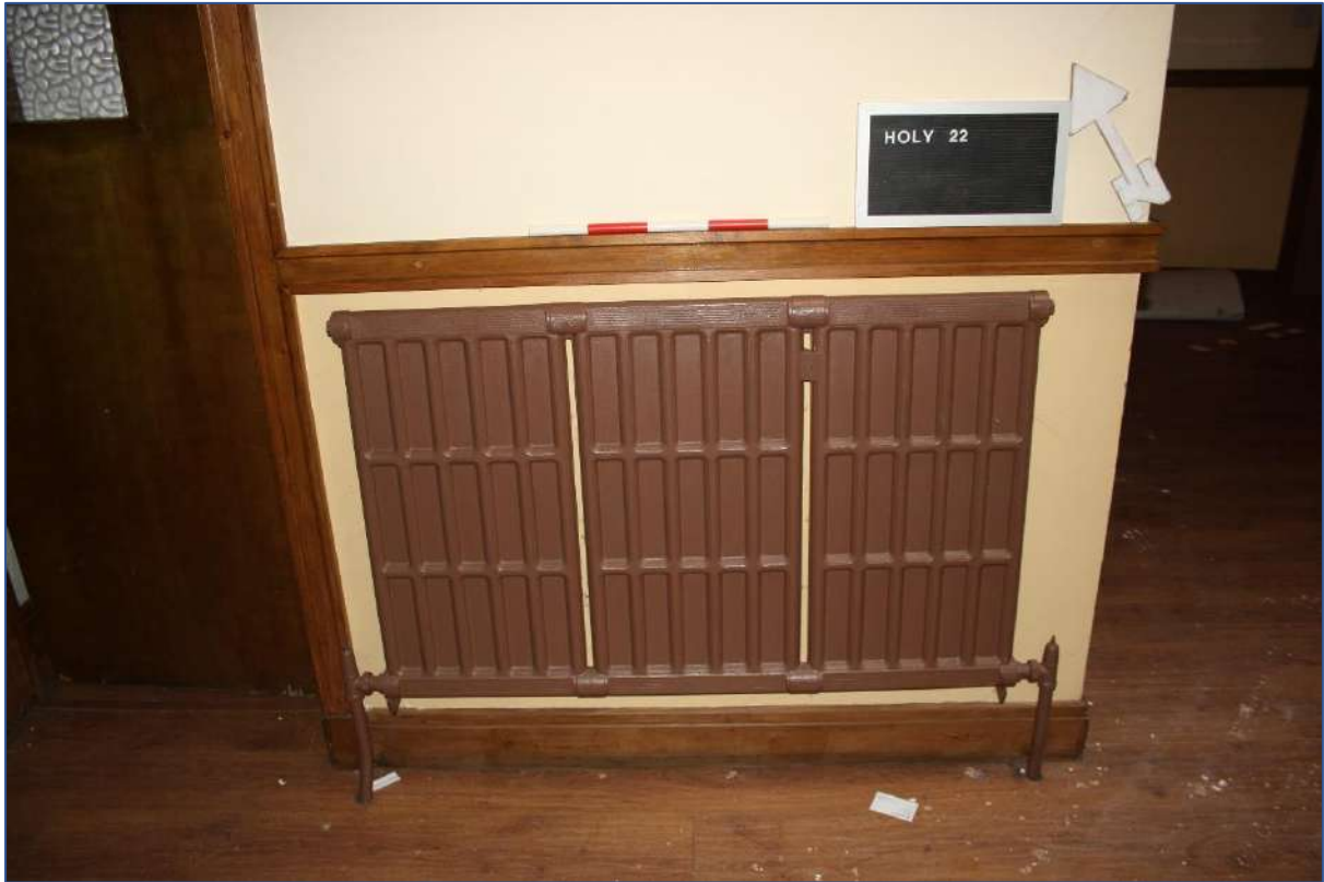
Plate 52: Radiator detail Room 5 looking E.
