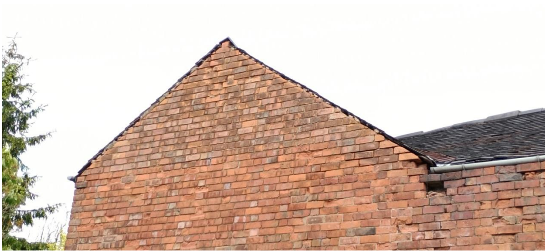
Photograph 1: External elevation showing brick gable end with weathering and potential access features.
