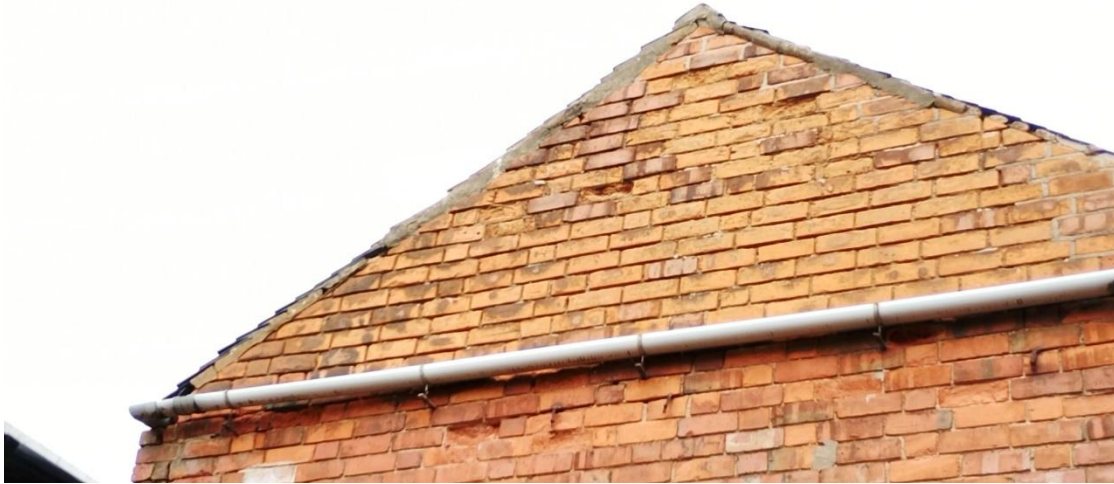
Photograph 9: Gable elevation showing weathered brickwork and roof junctions.
