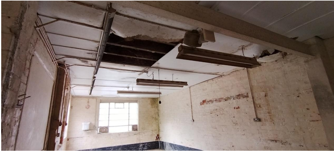
Photograph 5: Internal room showing damaged ceiling and exposed voids.
