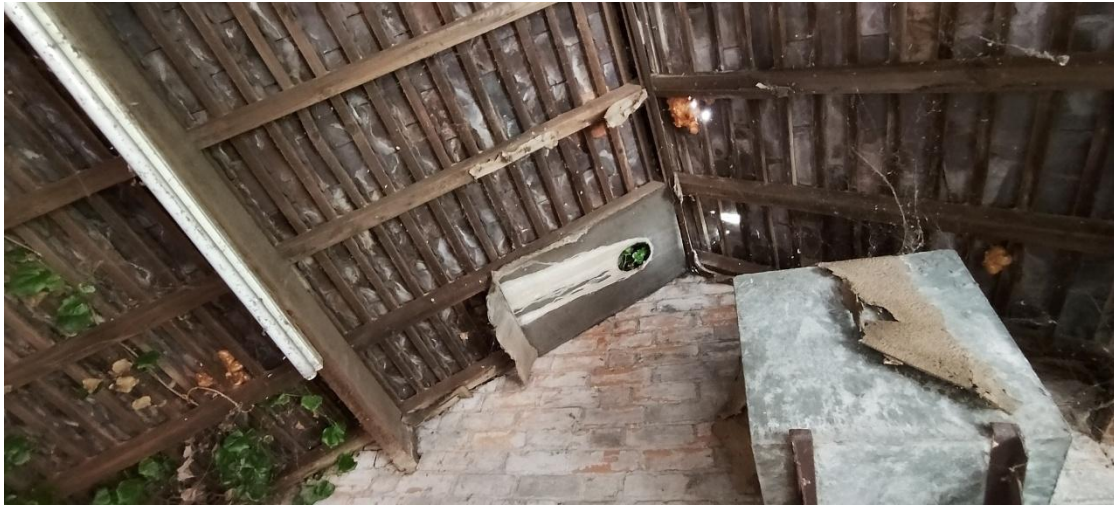
Photograph 3: Internal roof structure showing daylight ingress and potential access points.
