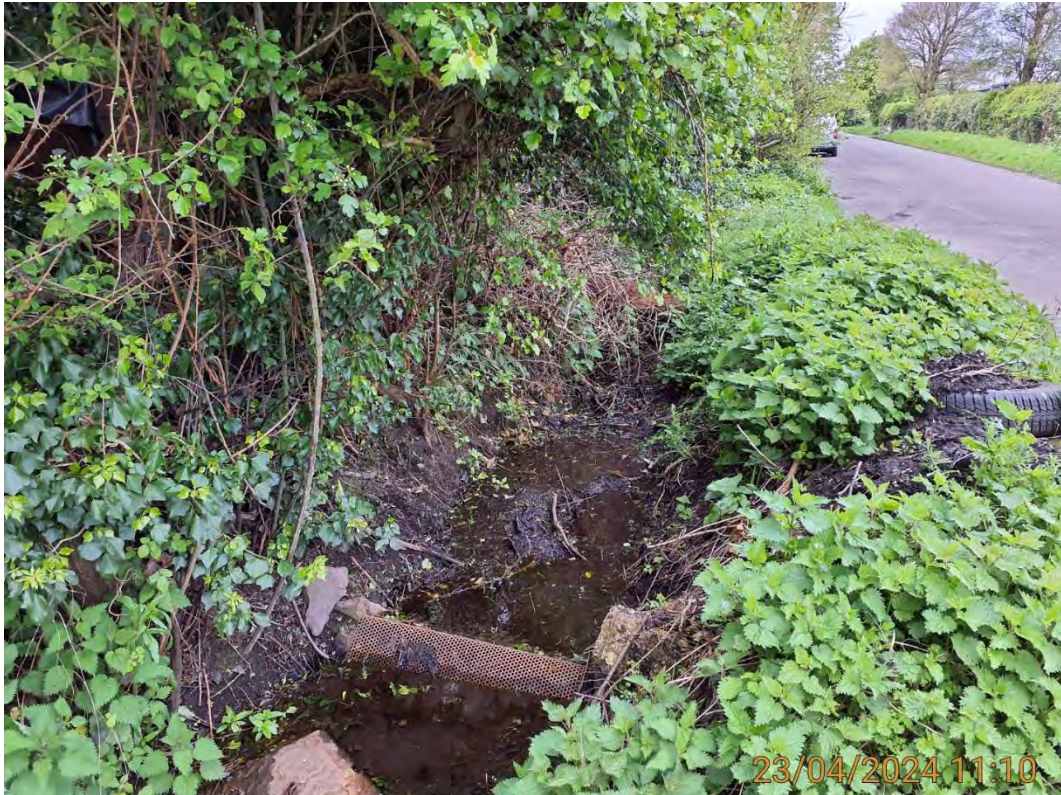
Plate 13 – Eastern end of the ditch on the northern boundary discharging into grill
