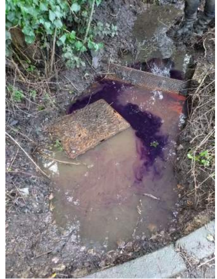
Ditch water dye goes to MH cover edge ii.JPG
