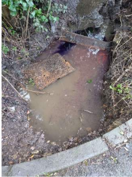
Ditch water dye goes to MH cover edge i.JPG
