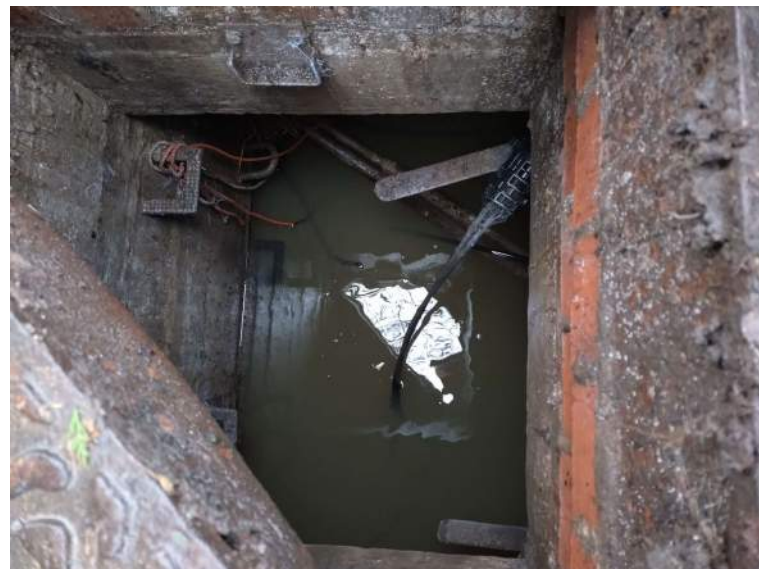
Cables cover opp ditch iv.JPG
