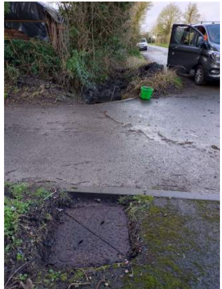
Cables cover opp ditch ii.JPG
