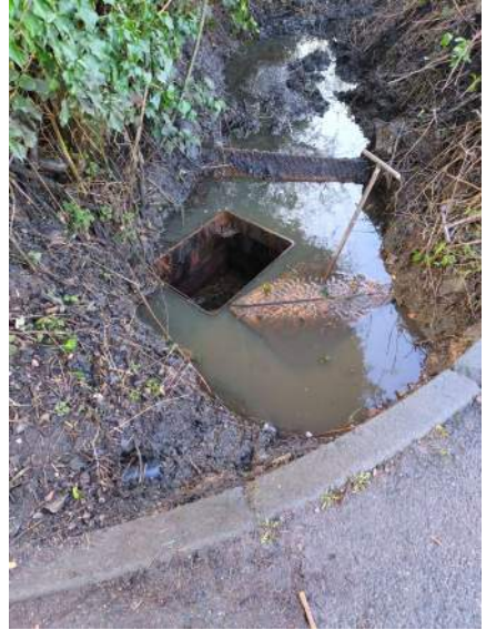
Ditch water level to MH edge.JPG
