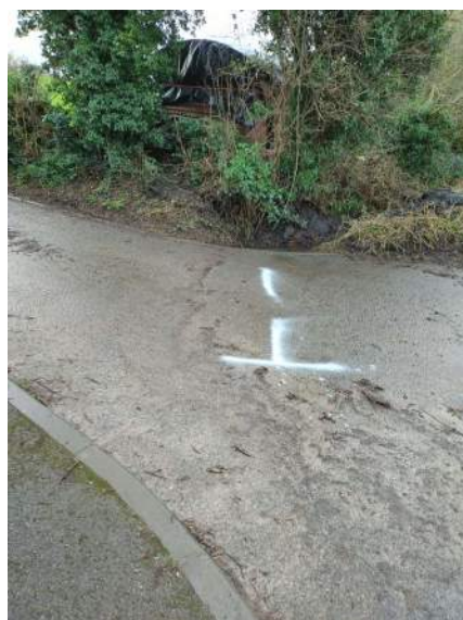
Line from MH blocked i.JPG
