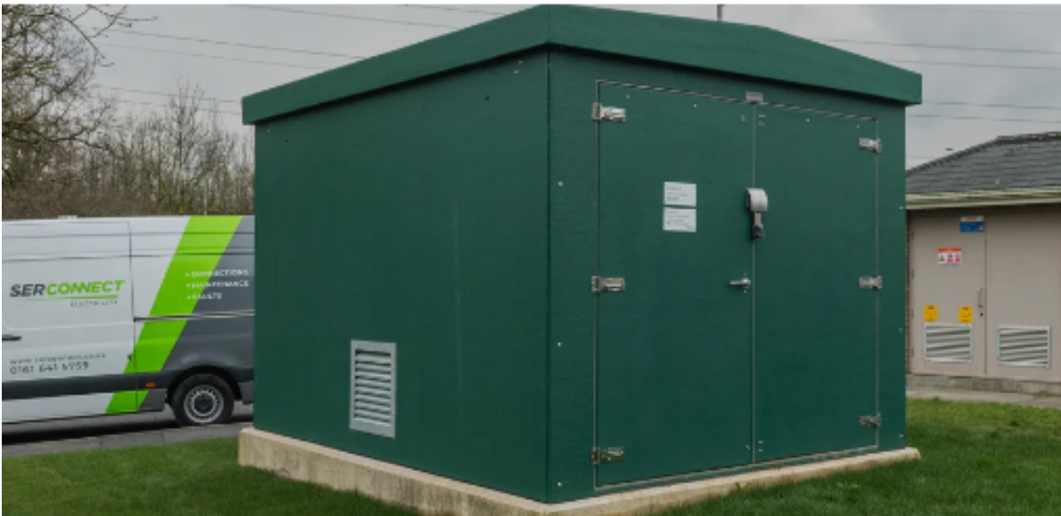
Photograph of typical substation and housing.
