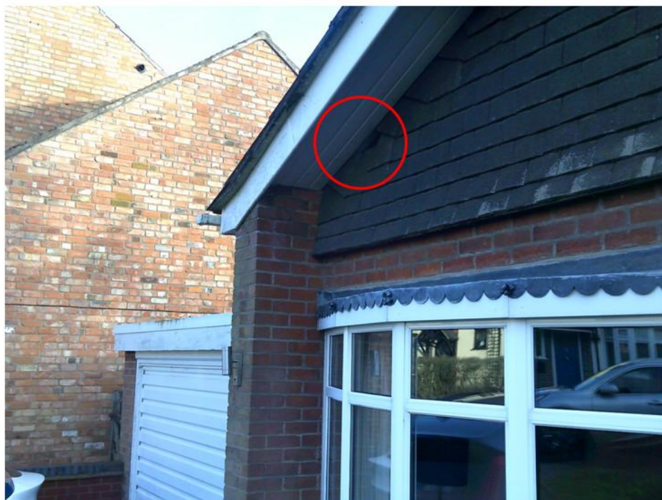
Gaps in front hanging tiles, endoscope inspected
