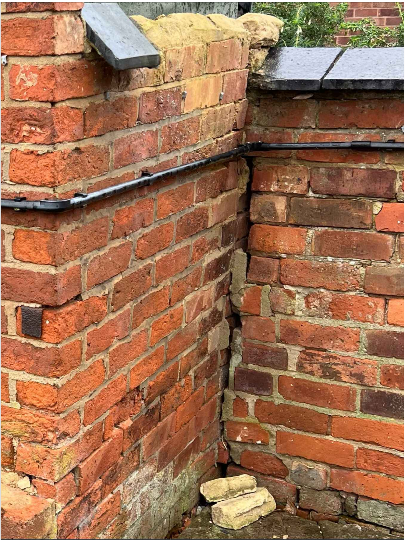
IMAGE 3 - SHOWCASES THE CONDITION OF THE WALL ON THE PATIO SIDE
