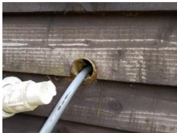
Plate A4.13: Example of hole in boards for pipes to enter building.
