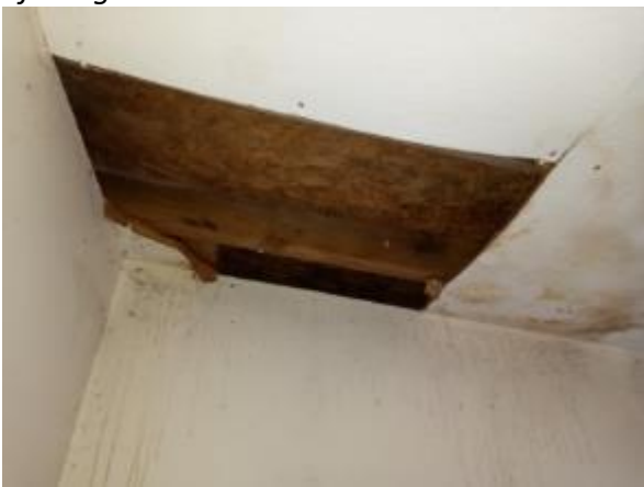
Plate A4.5: Example of missing ceiling panel.
