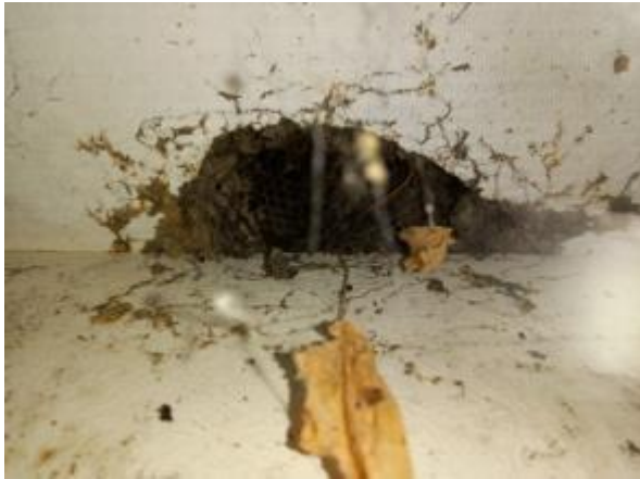
Plate A4.14: Hole in living room ceiling blocked by bees nest.
