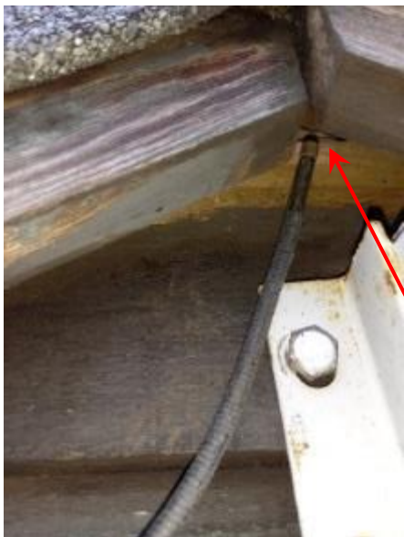
Plate A4.8: Gap at apex on west elevation – a possible access point for bats to enter the roof void.
