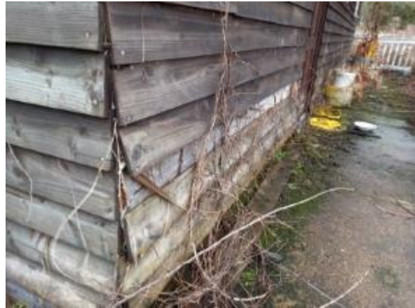
Plate A4.11: Example of minor peeling wooden cladding.
