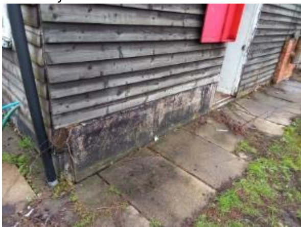
Plate A4.12: Missing boards on western elevation.
