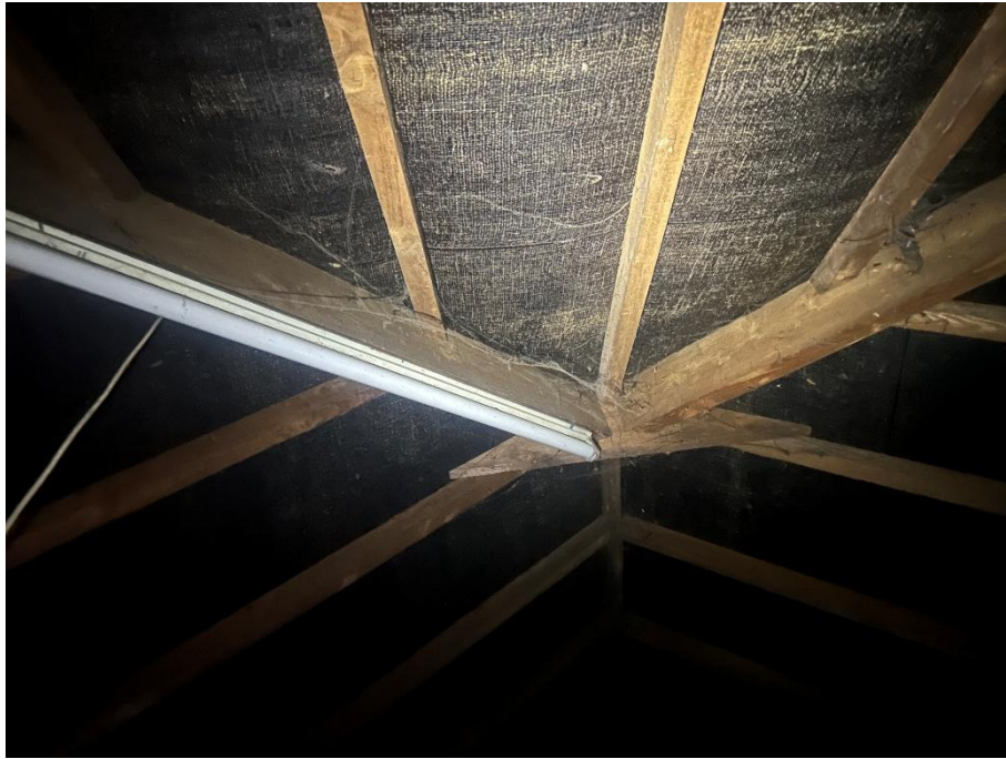
Photograph 10 – The internal loft space, showing high levels of cobweb cover
