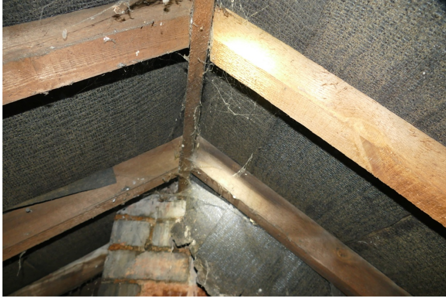
Photograph 6 – roof detail showing spider's webs.
