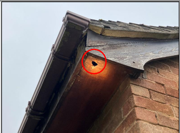
Figure 2. Exterior of B1, hole within the soffit board
