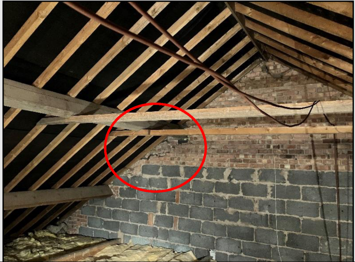
Figure 1. B1 cracks within the brickwork
