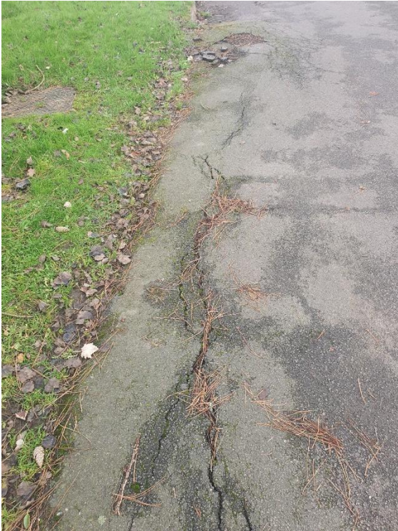
Damage to the adjacent road from tree roots.
