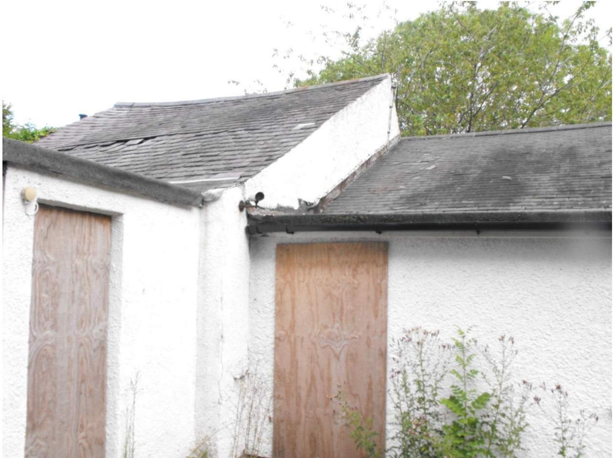
Slipped tiles rear dining
