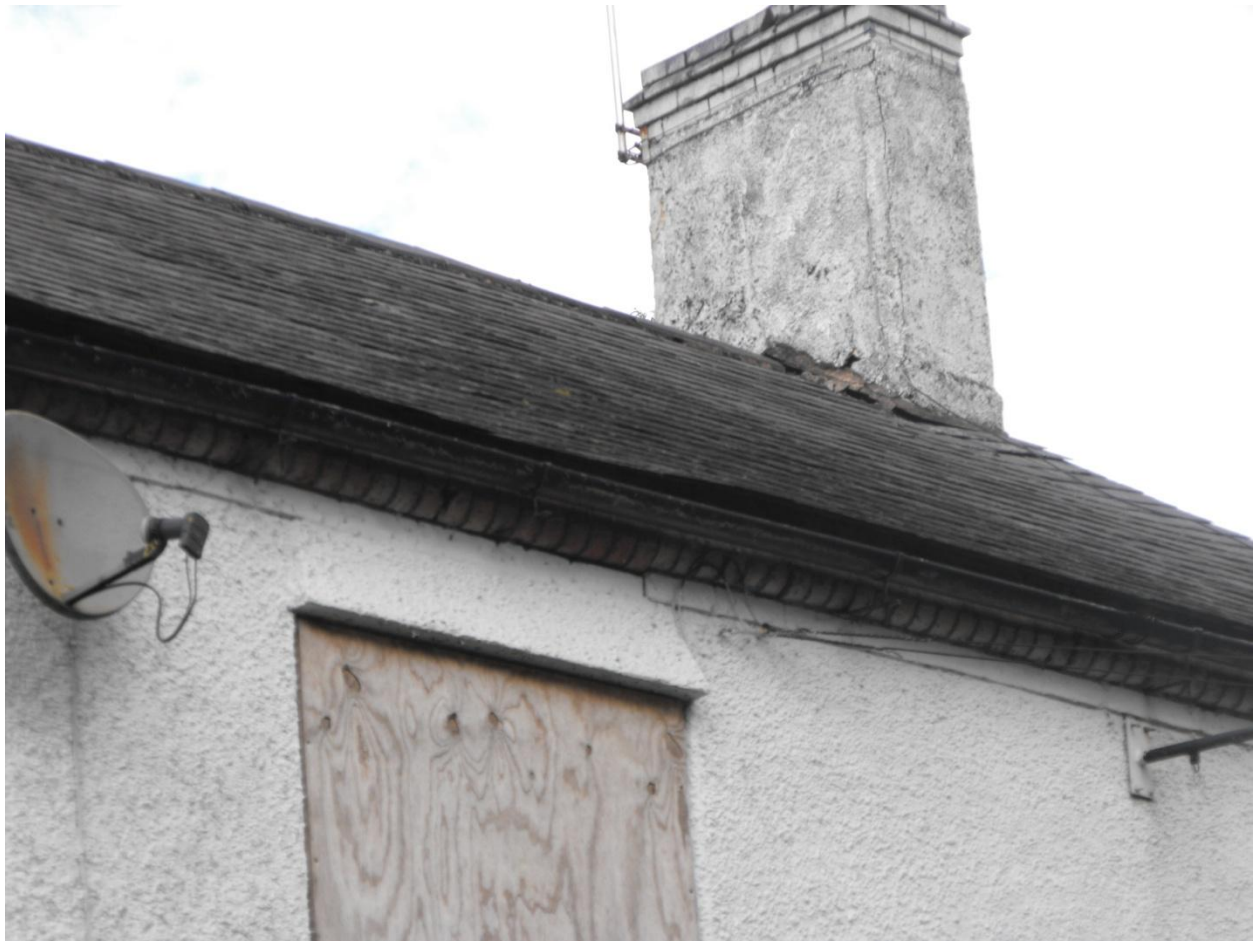
Missing mortar by chimney
