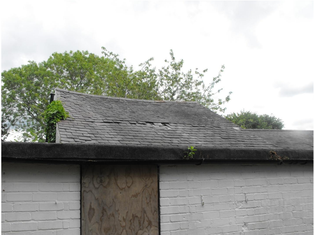
Slipped tiles on rear dining area
