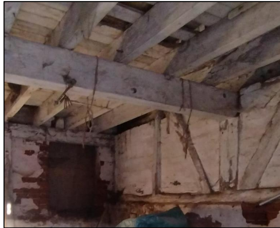
Photograph 6: Representative image of the cobwebbing of the ceiling structure in the barns lower level.
