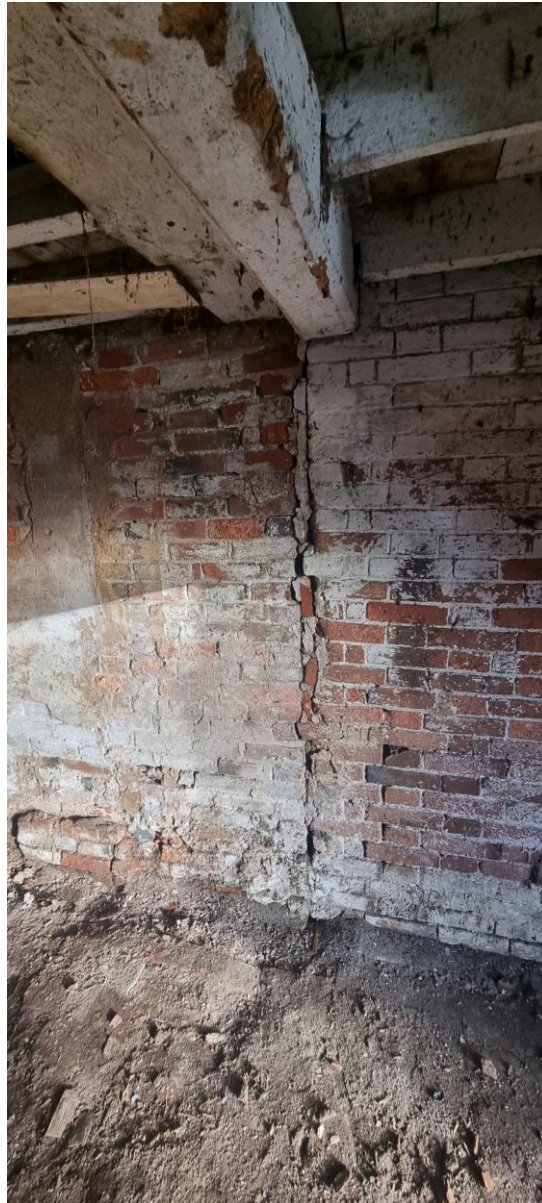
INTERNAL CRACKING TO MASONRY
