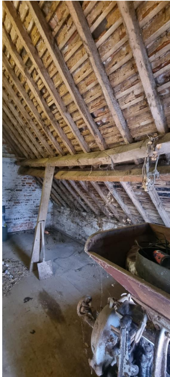
PURLINS WITH BOWING AND REPAIRS VISIBLE
