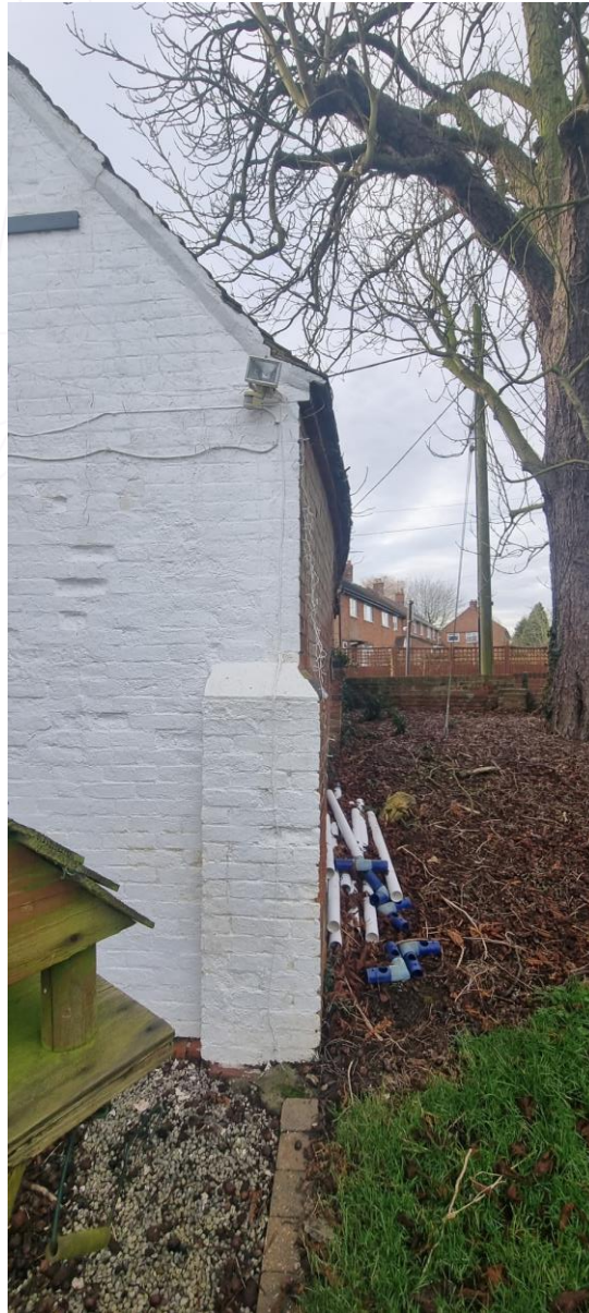
REAR WALL BULGING
