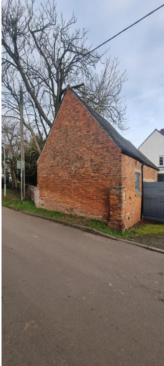
GABLE WITH SPALLED BRICKWORK
