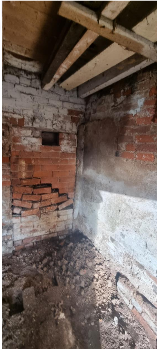
LOOSE BRICKS INTERNALLY AND CRACKING
