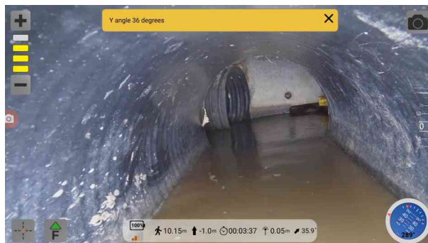
4, 00:01:39, 10.15 m Survey abandoned, LIMIT OF SURVEY DUE TO DIAMETER CHANGE , MH IN VIEW
