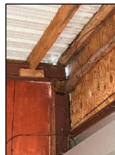
Opening into the building covered in cobwebs.
