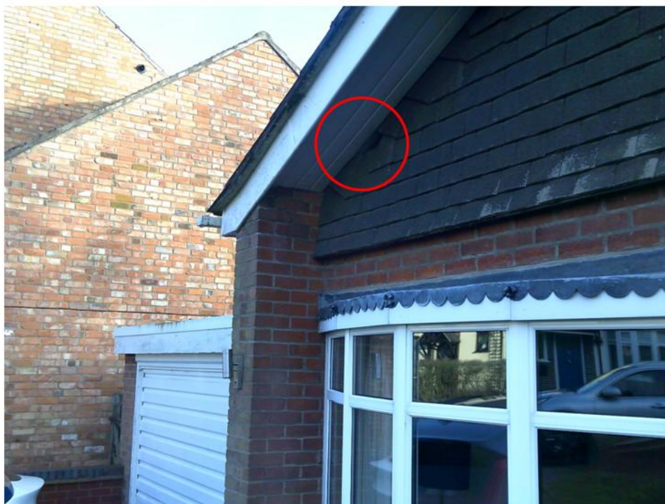
Gaps in front hanging tiles, endoscope inspected
