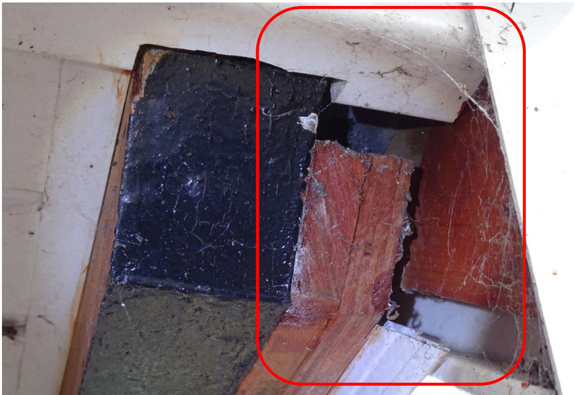
Image 2 – Gaps of adequate proportions to offer shelter/access opportunities for bats observed within the front eaves coverings of the property
