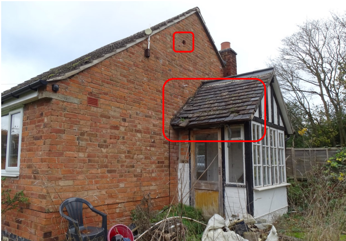
Image 3 – South facing elevation offering further gaps within the lower roof coverings and brickworks with likely access/shelter opportunities for bats
