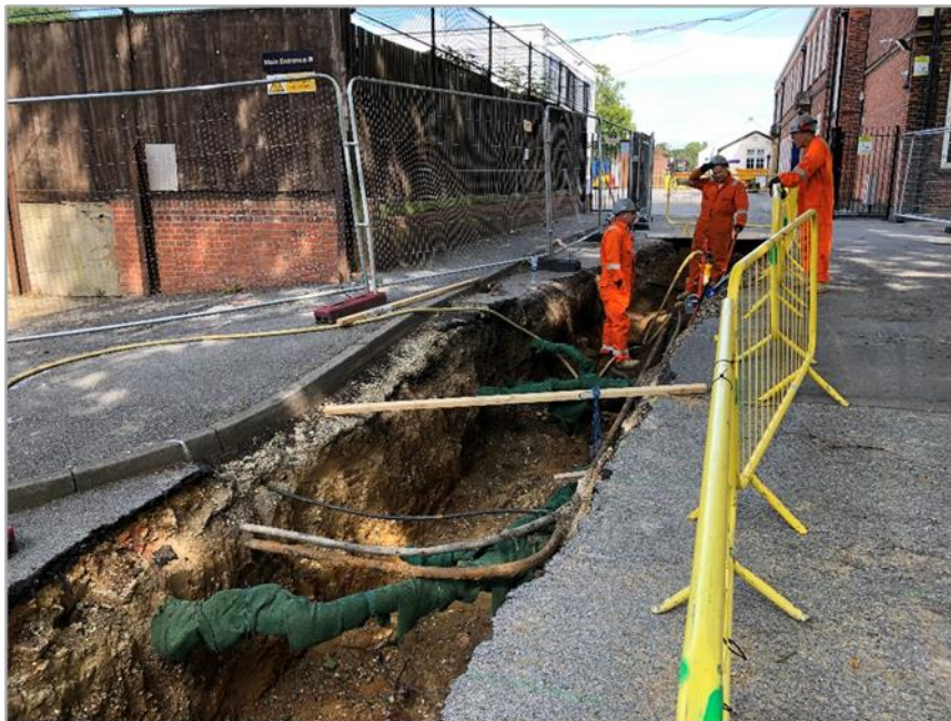
Figure 5 – Retained roots in service trench.
