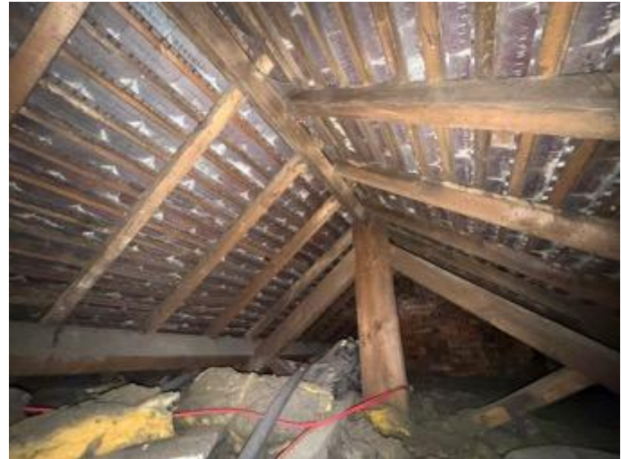
Internal area of B1
