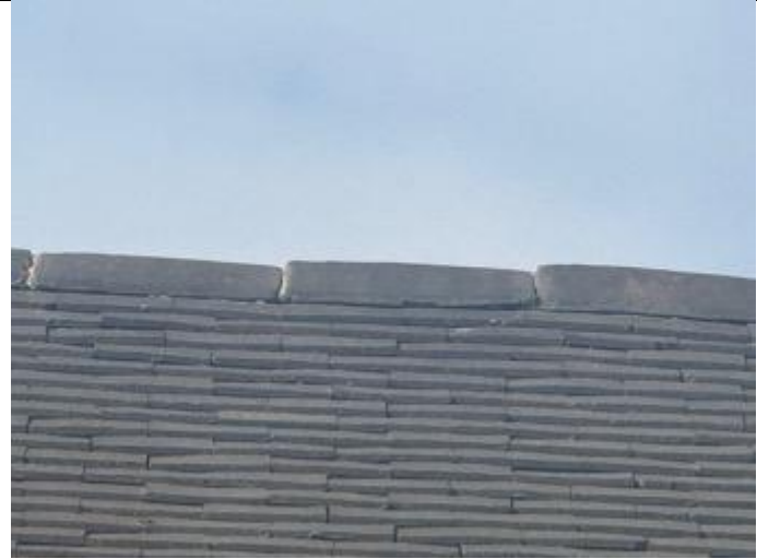
Example of gaps within roof structure of B1
