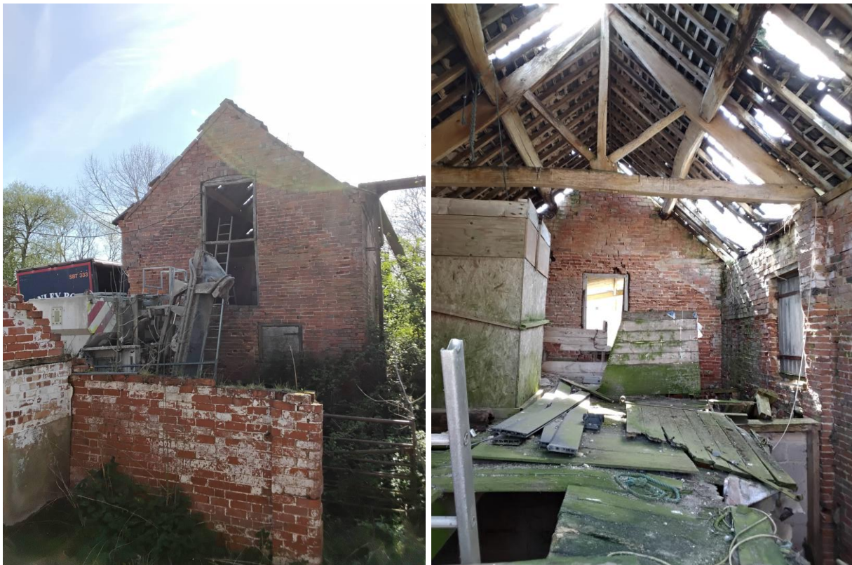
Photos 1 and 2. Dilapidated old brick buildings, the exterior (left image) and interior (right image)
