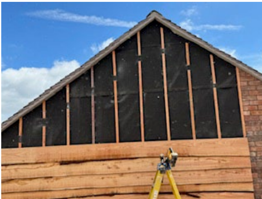
Waney edge cladding and gaps in timber battens on western elevation.
