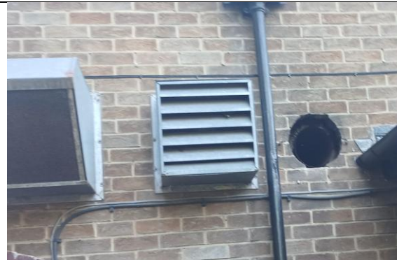
Figure 9 – large hole associated with old vent
