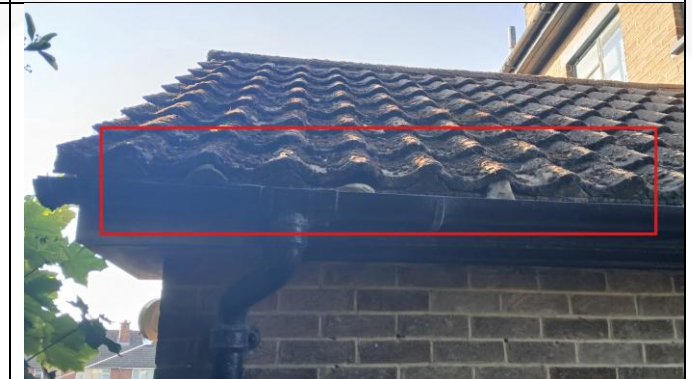
Figure 10 Minor gaps associated with bottom course of tiles on south eastern elevation of southwestern extension
