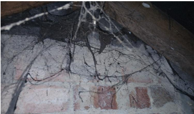
Figure 5 – Dense cobwebbing at gable apex
