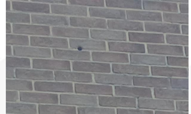
Figure 7 – hole in gable southeast elevation
