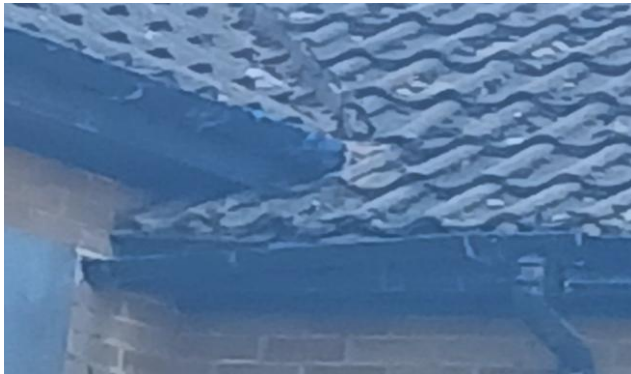
Figure 8 – minor raised tiles at valley on south eastern elevation
