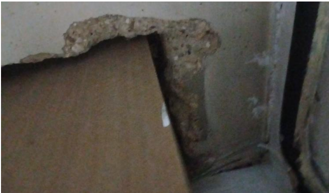
Figure 5 – internal cellar crevice network
