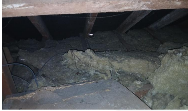
Figure 6 – Light ingress at eaves
