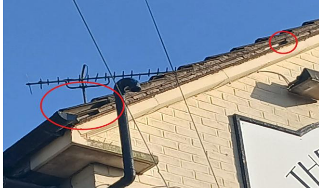
Figure 6 – verge gaps northwest elevation
