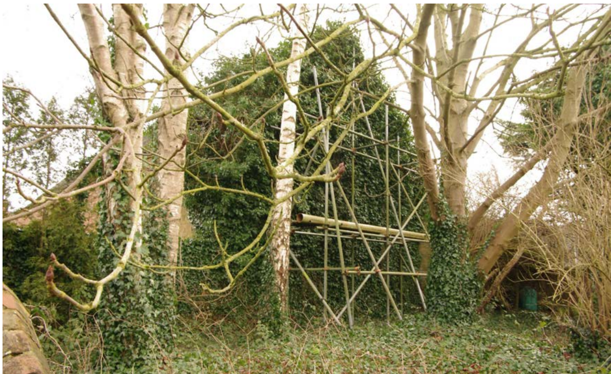
Figure 30: Threshing barn. South-west facing gable end Looking east. Hardly any brickwork was visible during the survey. The scaffolding suggests a poor and unstable condition so no attempt was made to remove the vegetation
