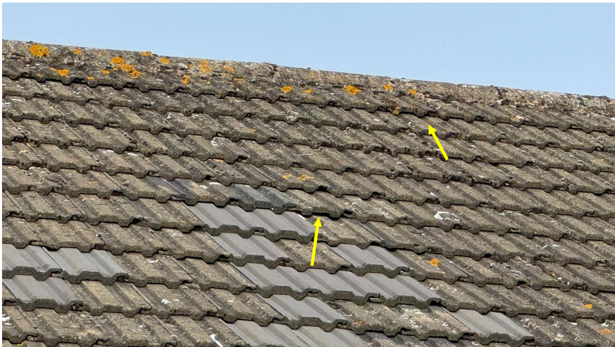
Photograph 10: The slightly lifted roof ties, which are otherwise well fitted, including sections of replaced tiles.
