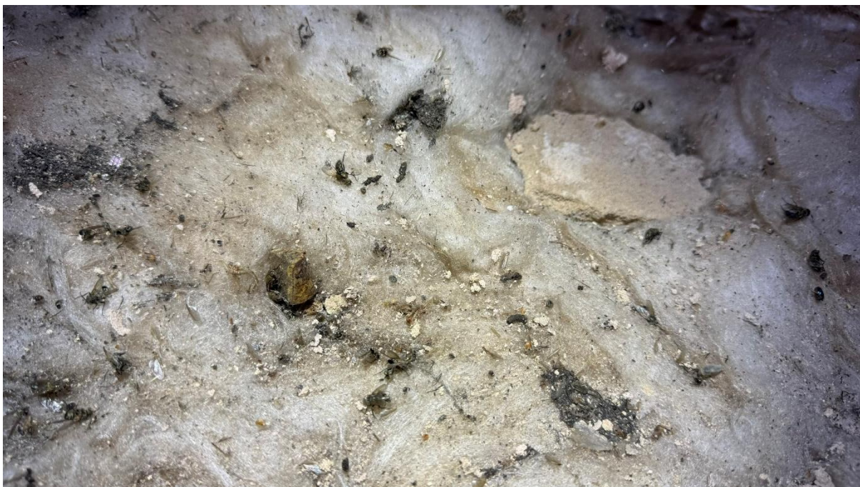
Photograph 4: The small aggregation of droppings located at the eastern end of the roof void, below the ridge.
