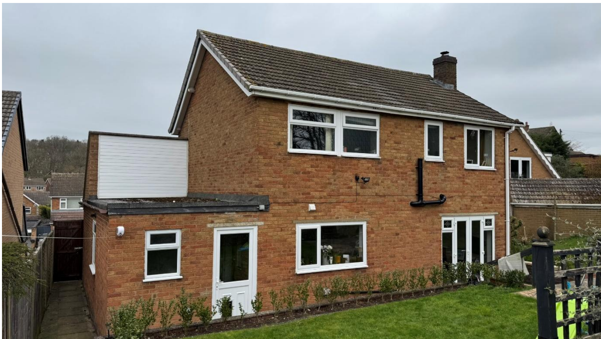
Photograph 2: The dwelling, taken from the south-west, showing the uPVC weatherboarding on the rear of the roof covering over the garage.
