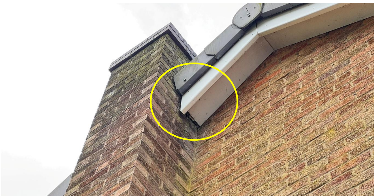
Photograph 8: The gap behind the soffit box, adjacent to the chimney, which is the primary roost feature/access feature.
