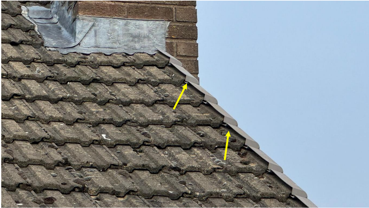
Photograph 9: Evidence of the gaps behind the verge capping.
