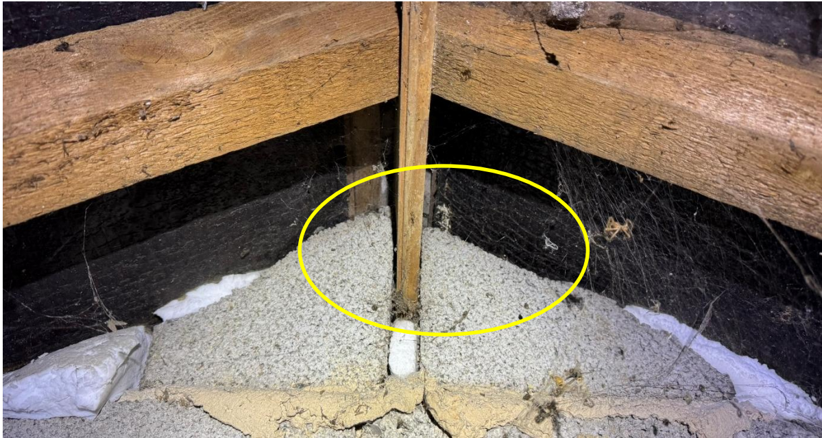
Photograph 7: The small gaps over the internal gable which may provide an access point for bats.
