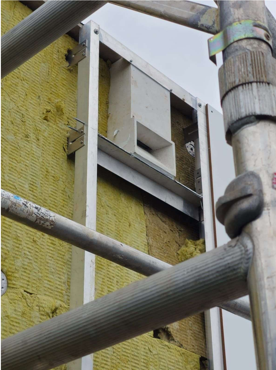
FIGURE 9 - X1 BAT BOX INSTALLED ON SOUTH ELEVATION
