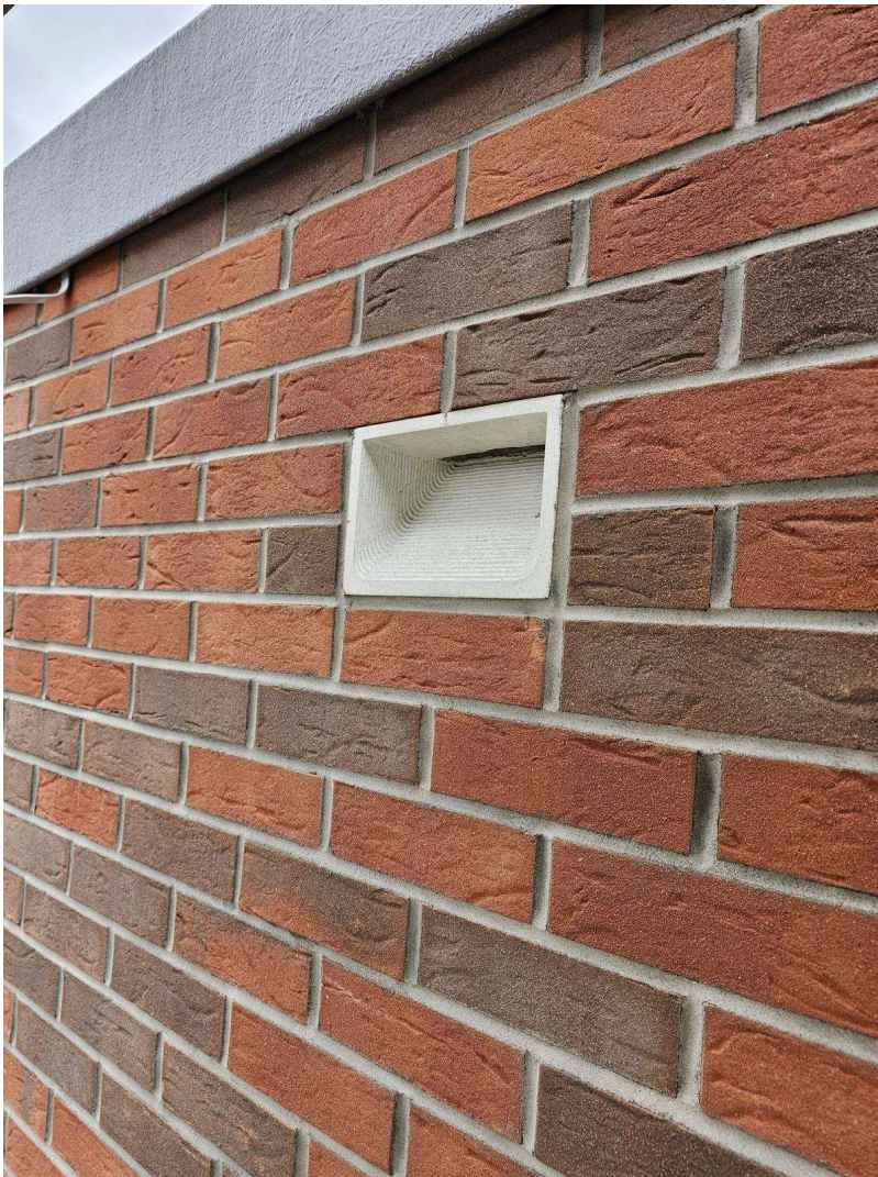
FIGURE 6 - X1 BAT BOX INSTALLED ON NORTH ELEVATION
