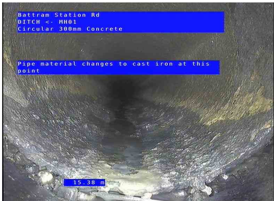
DITCHX_9ecd039f-0d38-4e0e-8242-dd12647defbf_20250903_081127_438.jpg, 00:01:54, 15.38 m Pipe material changes to cast iron at this point
