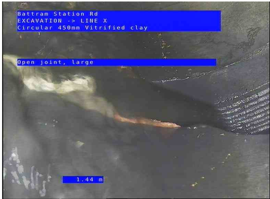
EXCAVATIONX_7ea59fd8-fb10-4512-b408-4e7c7cde6ac6_20250903_104613_004.jpg, 00:00:27, 1.44 m Open joint, large
