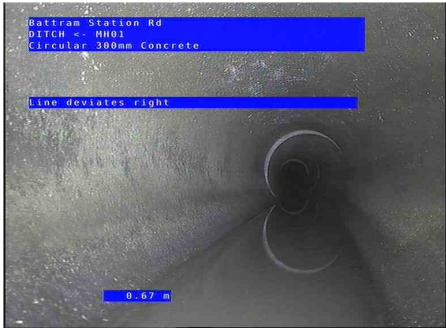
DITCHX_5214dd6a-503b-43d4-9791-001bcfb0fe31_20250903_080956_133.jpg, 00:00:33, 0.67 m Line deviates right
