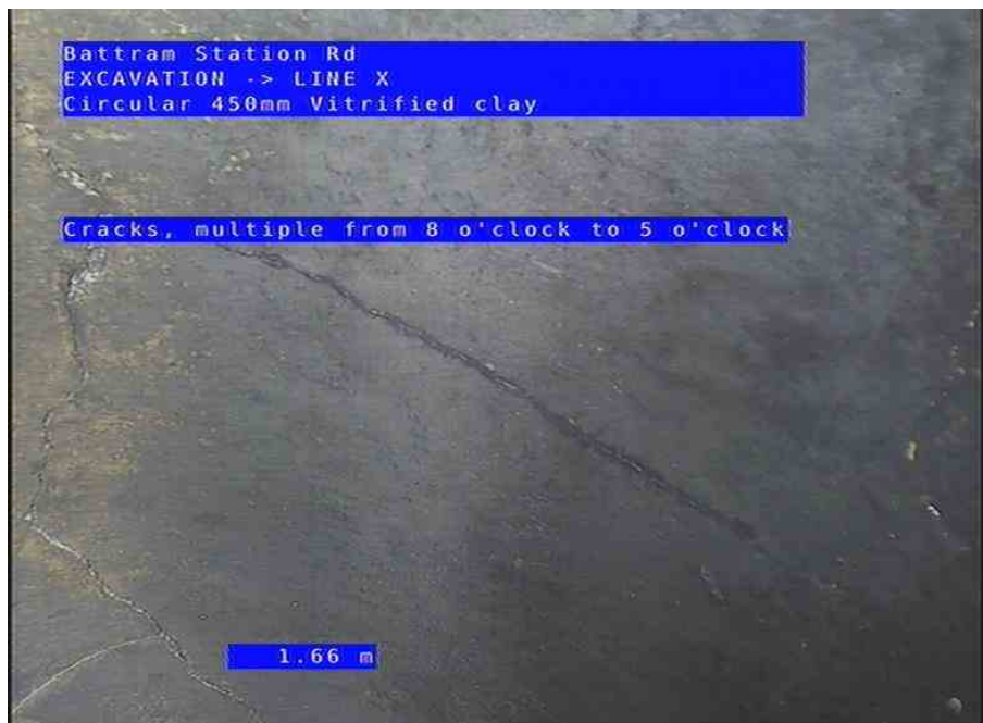
EXCAVATIONX_5e9b7dfb-c590-4c6a-b6b5-43c09af10d88_20250903_104642_625.jpg, 00:00:49, 1.66 m Cracks, multiple from 8 o'clock to 5 o'clock
