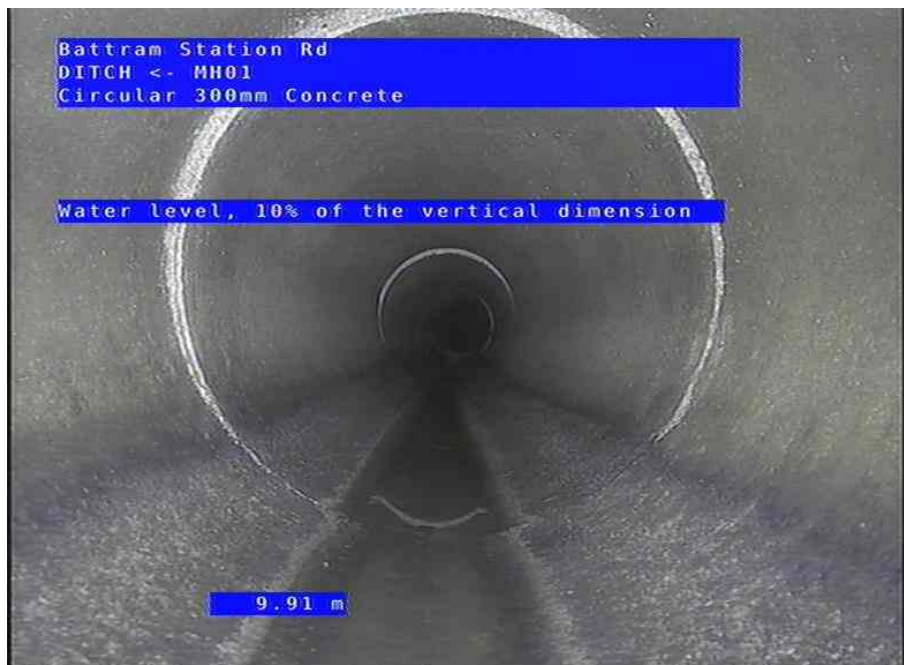
DITCHX_8d891bd5-cded-4226-969d-6ffb089eb3f_20250903_081033_938.jpg, 00:01:08, 9.91 m Water level, 10% of the vertical dimension
