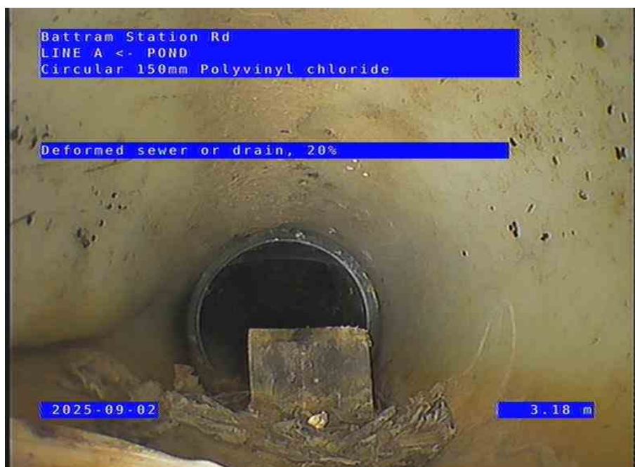
LINE A X_f8dc6610-d613-44ac-b0fa-f0f89af9d991_20250902_102058_725.jpg, 00:00:35, 3.18 m
