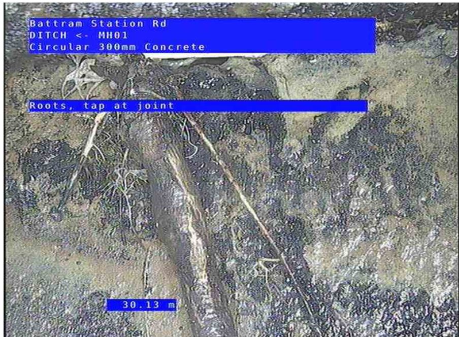
DITCHX_2b29cf83-7194-4120-bf1b-24b736061227_20250903_081346_907.jpg, 00:03:43, 30.13 m Roots, tap at joint
