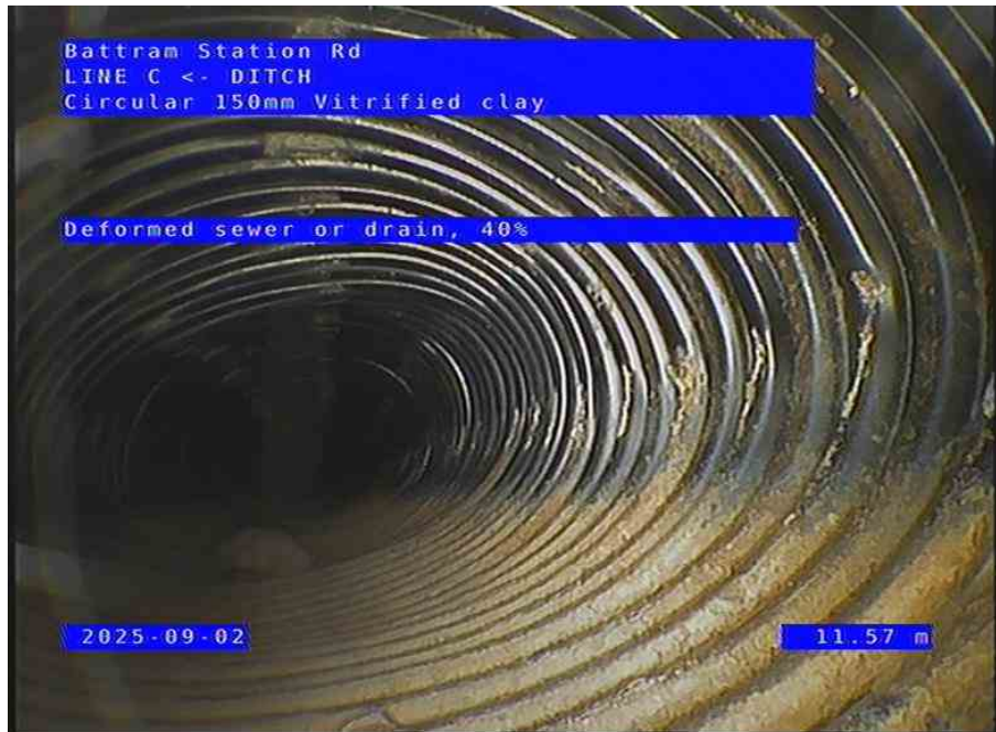
LINE C X_5404a792-ada1-4d04-9347-c4bafec37514_20250902_112843_198.jpg, 00:01:17, 11.57 m Deformed sewer or drain, 40%
