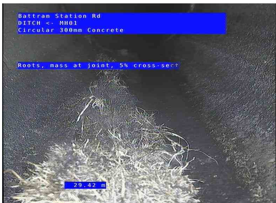
DITCHX_70383fd2-f27f-4e59-bf71-0c6ca39322c7_20250903_081328_845.jpg, 00:03:29, 29.42 m Roots, mass at joint, 5% cross-sectional area loss
