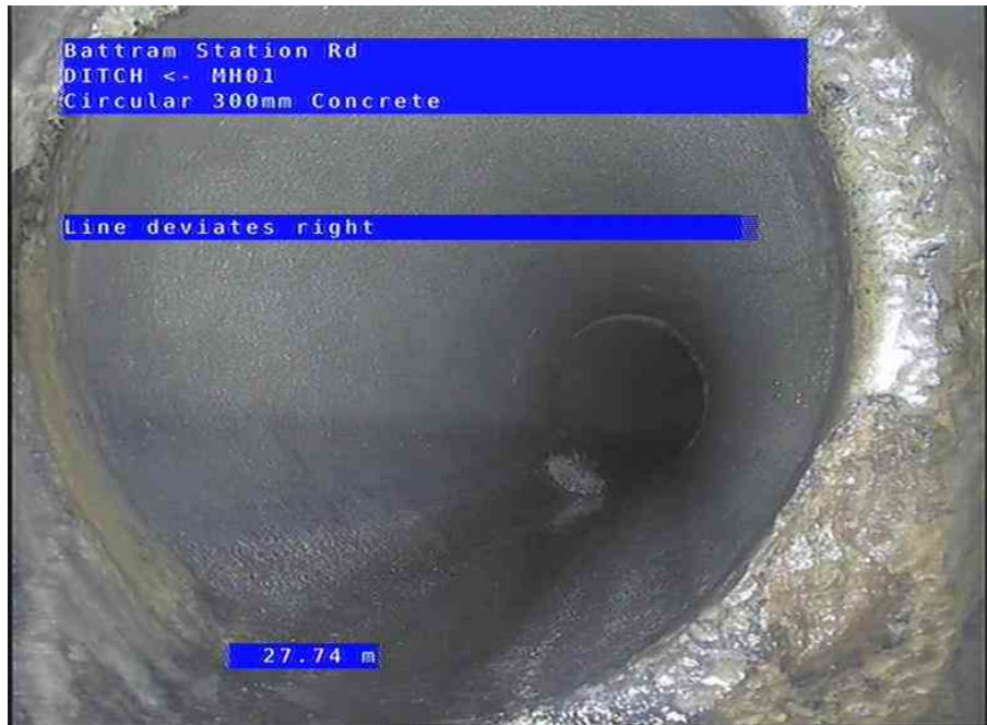
DITCHX_9f341506-a52d-4792-af79-6ab0f0f00e93_20250903_081311_390.jpg, 00:03:18, 27.74 m Line deviates right
