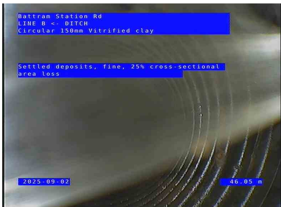
LINE B X_4f7ee2b8-4565-4925-9930-c6a7cf788497_20250902_112202_988.jpg, 00:03:48, 46.05 m Settled deposits, fine, 25% cross-sectional area loss
