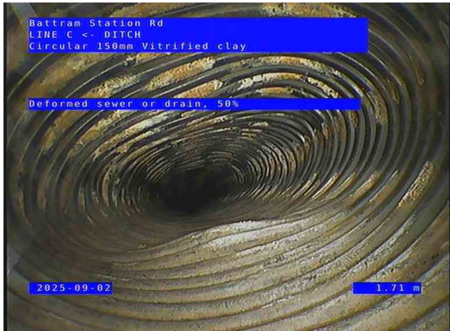
LINE C X_f2df2e9e-1e01-4f3a-bd2c-fee4eb057bf0_20250902_112746_685.jpg, 00:00:28, 1.71 m Deformed sewer or drain, 50%
