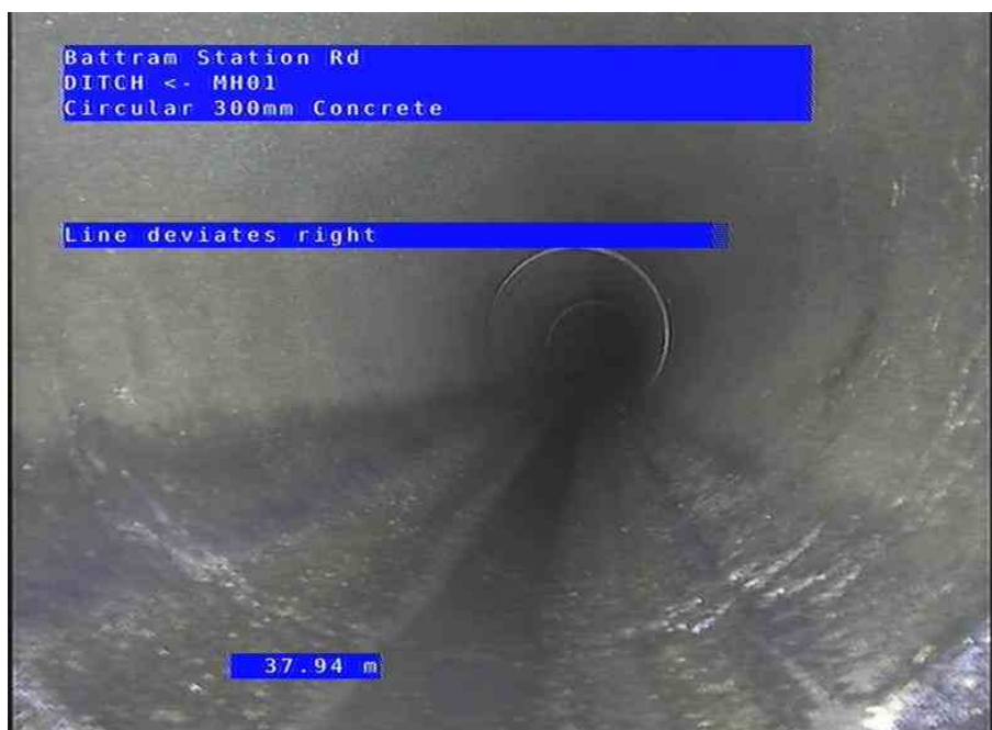
DITCHX_ddc7877f-1efc-4e29-92b3-76e5e1644646_20250903_081420_974.jpg, 00:04:11, 37.94 m Line deviates right
