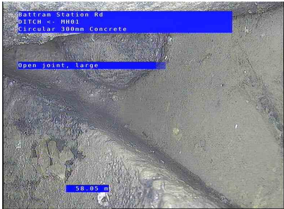
DITCHX_a44096a9-02a8-46a0-a2e5-1f4cf2b29d78_20250903_081547_857.jpg, 00:05:35, 58.05 m Open joint, large
