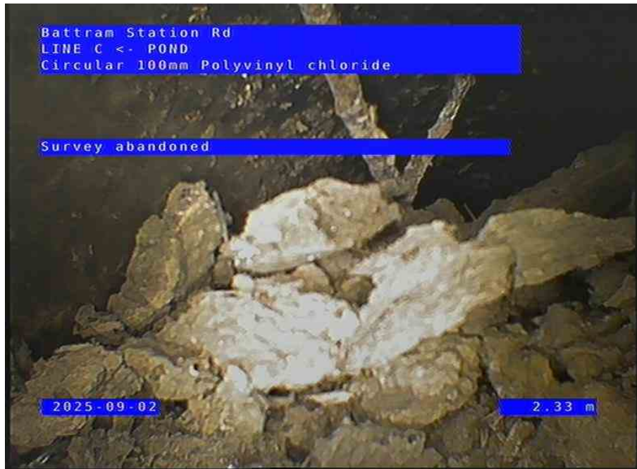
LINE C X_3e150bce-d529-4956-879b-990377a62418_20250902_104549_988.jpg, 00:01:21, 2.33 m Survey abandoned
