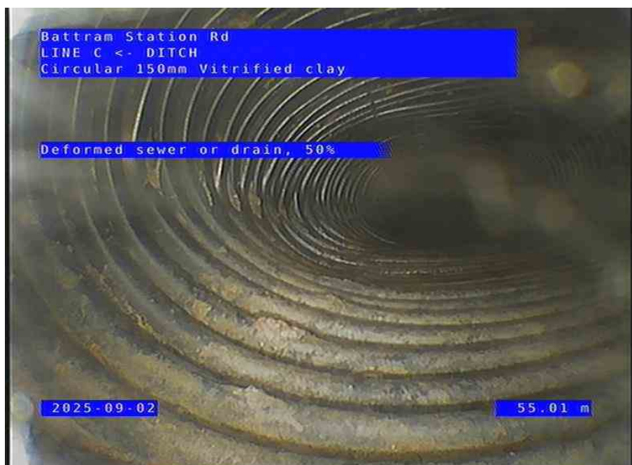
LINE C X_afbd2fc8-7777-4fd3-a672-df75609fc39e_20250902_113053_259.jpg, 00:03:16, 55.02 m Deformed sewer or drain, 50%
