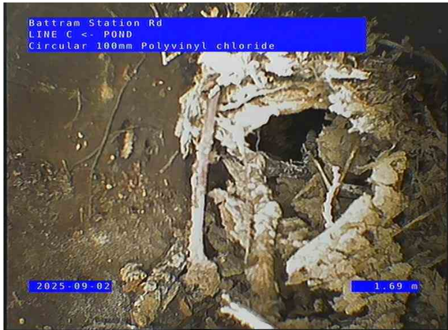
LINE C X_f81d3e96-b997-4124-8110-9d398f2f7348_20250902_104510_719.jpg, 00:00:47, 1.69 m
