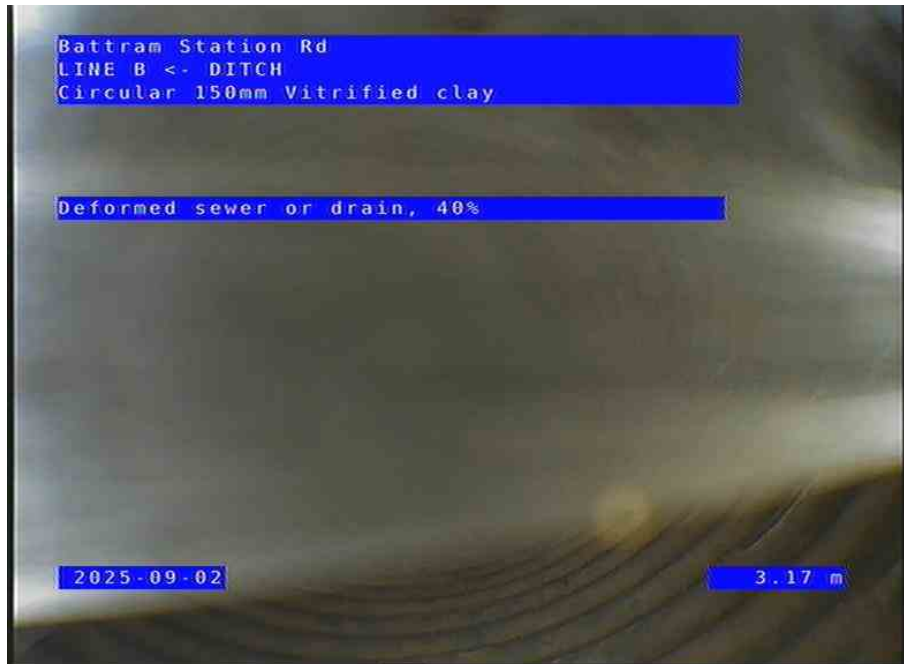
LINE B X_771ba19a-6b3c-43cf-8cca-d9eadca2e894_20250902_111903_661.jpg, 00:00:59, 3.16 m Deformed sewer or drain, 40%
