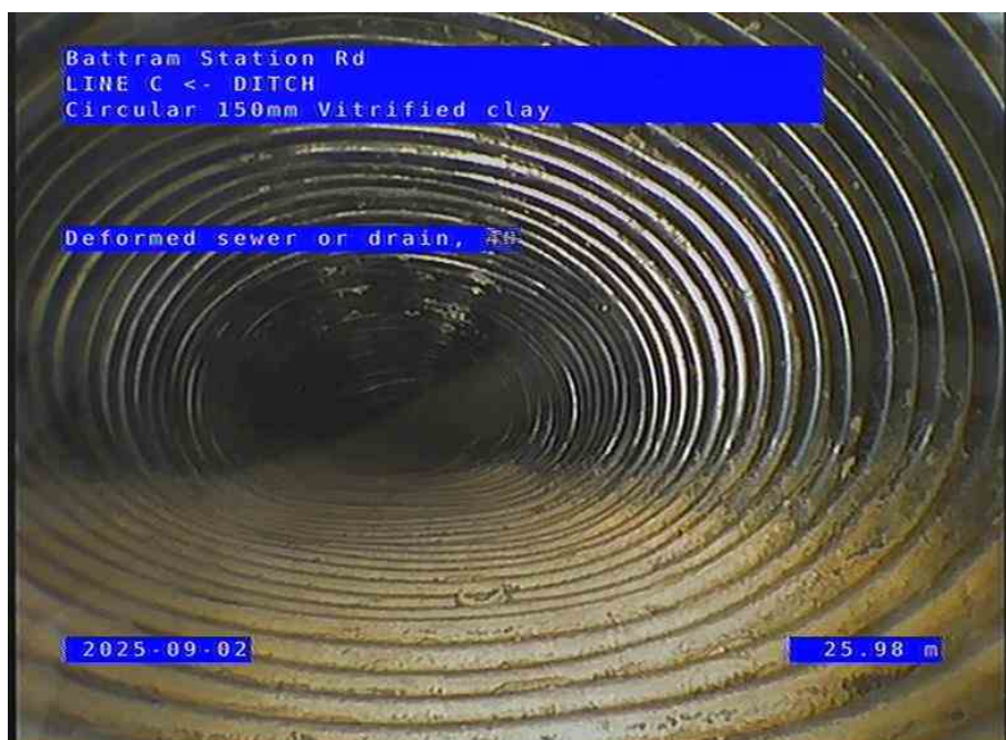
LINE C X_4ca82f9c-9923-4f92-860d-def0f38eb5af_20250902_112929_611.jpg, 00:01:59, 25.98 m Deformed sewer or drain, 40%
