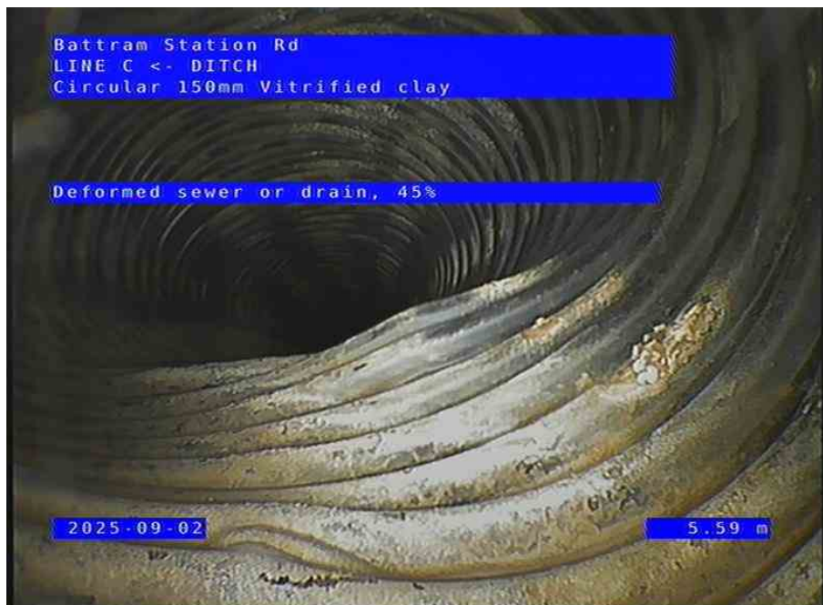
LINE C X_febc130c-1b4c-4cc0-a10a-1be522bb8f7a_20250902_112815_746.jpg, 00:00:52, 5.59 m Deformed sewer or drain, 45%
