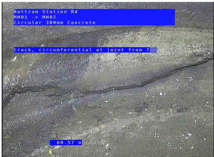
MH01X_e2de7cd5-0c3f-450e-82bd-aa9b224ed0d7_20250902_143521_145.jpg, 00:04:25, 60.57 m Crack, circumferential at joint from 7 o'clock to 11 o'clock
