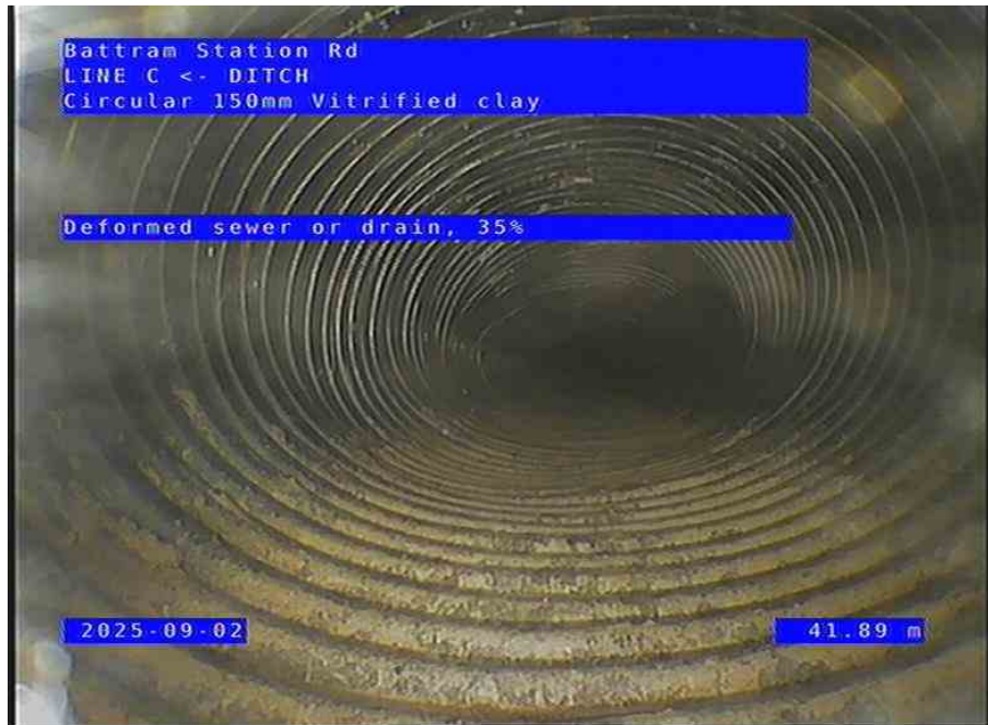
LINE C X_3f2f0429-994f-4ed7-a8d9-6644d562461f_20250902_113012_819.jpg, 00:02:38, 41.89 m Deformed sewer or drain, 35%
