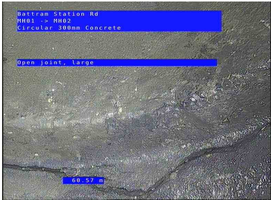
MH01X_b1033ddd-e303-4c28-849f-f78511d7cffd_20250902_143442_786.jpg, 00:04:02, 60.57 m Open joint, large
