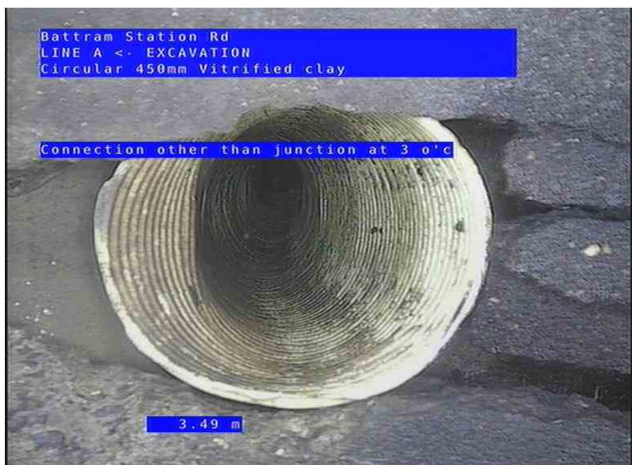
LINE A X_b0051871-698b-426b-9526-584446dd0b9e_20250903_105707_786.jpg, 00:00:26, 3.49 m Connection other than junction at 3 o'clock, 100mm dia
