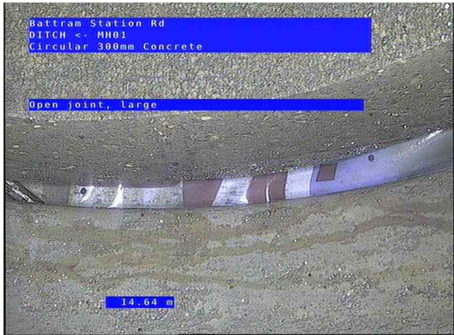
DITCHX_92cc8cd6-0789-4405-9870-a056ffe9a40a_20250903_081112_780.jpg, 00:01:44, 14.64 m Open joint, large
