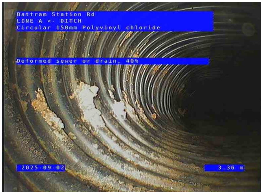
LINE A X_5a729ba0-b98f-47c8-b445-d26585673884_20250902_111436_516.jpg, 00:00:28, 3.36 m Deformed sewer or drain, 40%
