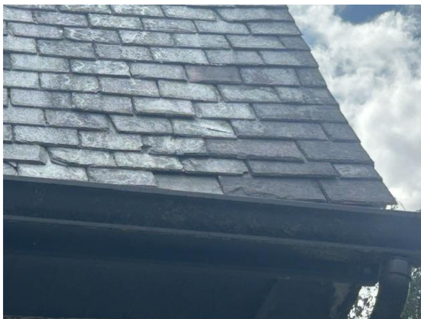
Figure 5 – Extent of gaps in tiles viewed on B1
