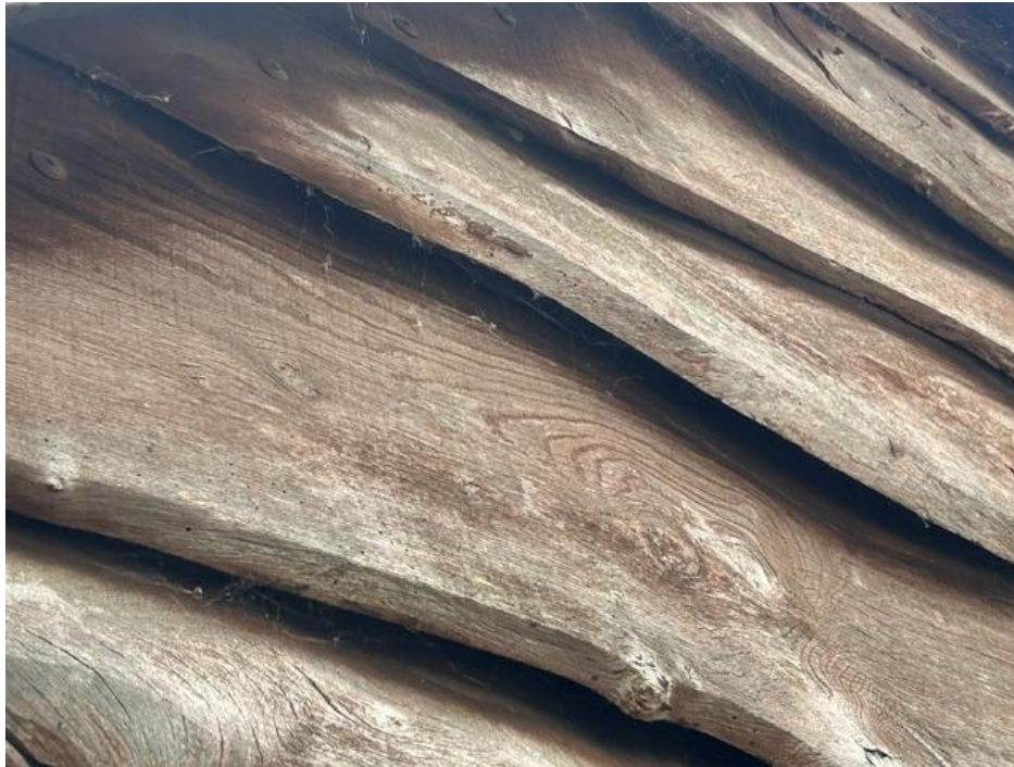
Figure 12 – Lifted cladding on B2
