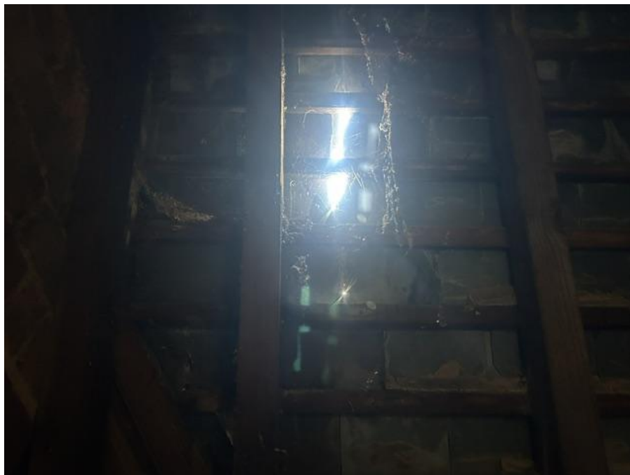
Figure 11 – Light ingress seen in loft space of B1
