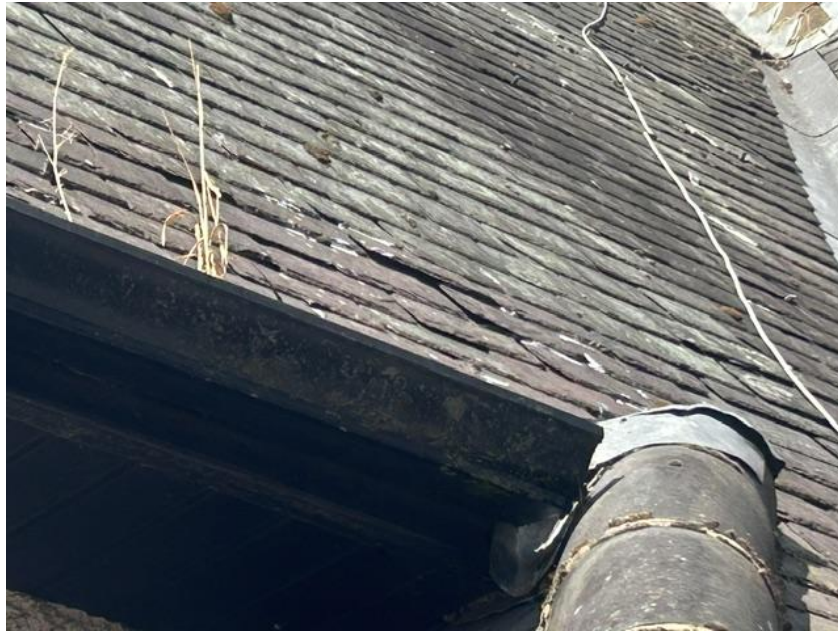
Figure 6 – Extent of gaps in tiles viewed on B1
