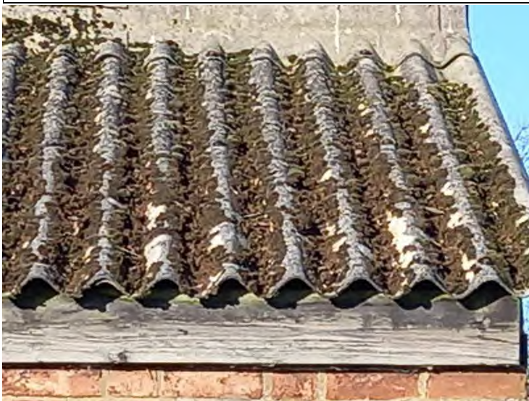
Photo 5—Barn roof possibly constructed out of asbestos containing materials.
