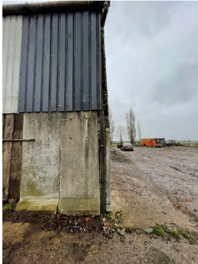
Figure 8: Barn A - Impacted column at the front left hand side corner of the building
