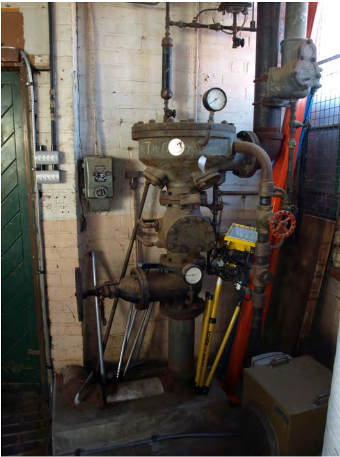
Plate 41: Mather and Platt Sprinkler system
