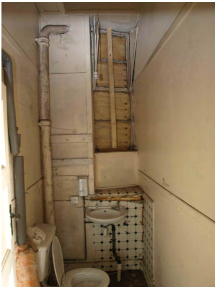
Plate 30: Toilet built into angle over carriageway
