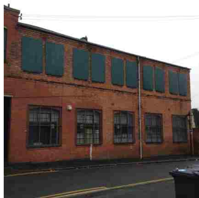
8 original factory typical Victorian character - very poor condition and repairs are no longer viable - the local authority accepted as part of the previous application that demolition of this building would be acceptable
