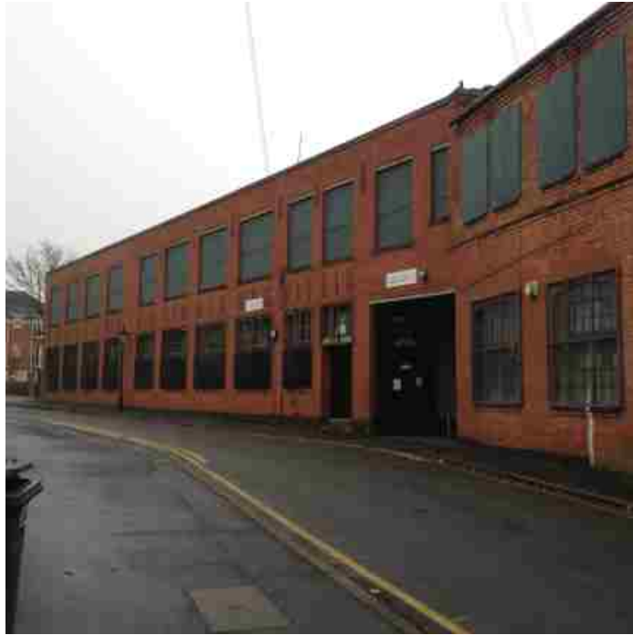
7 later factory building with flat roof behind parapet extended off original factory - ground floor currently in use but first floor is unlettable and in need of significant repair
