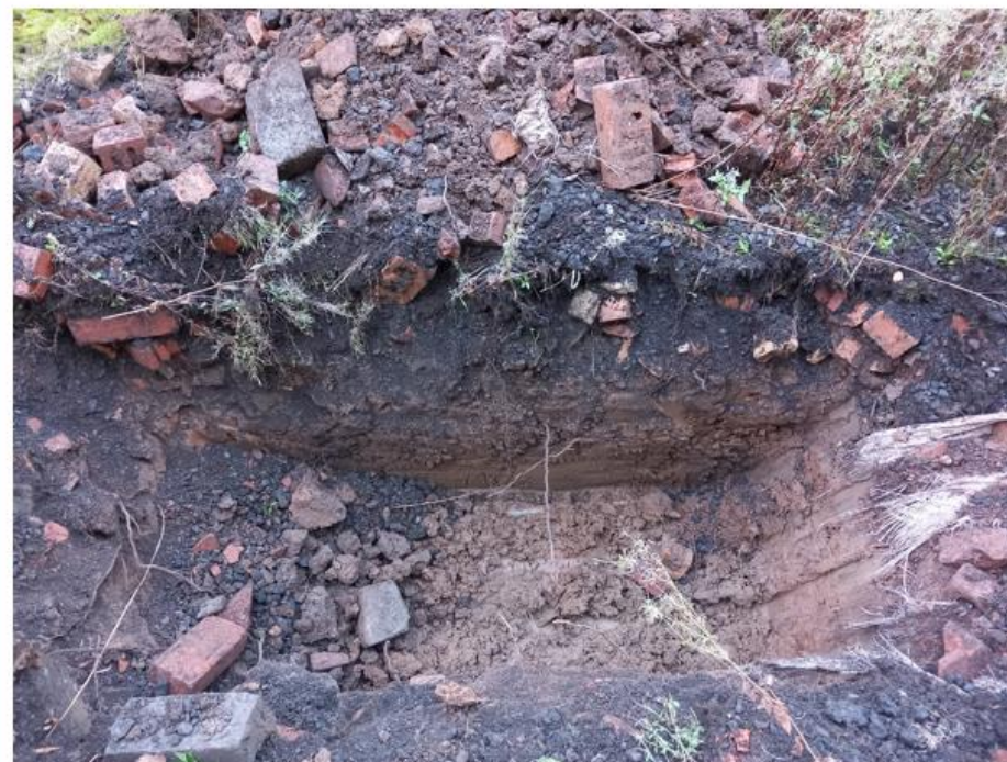
Photo No.6: TP03 pit sides and base showing made ground atop made ground sand infill (service strike at 0.80m – water)
