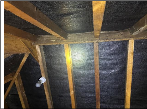
Photo 5 Heavily cobwebbed roof void
