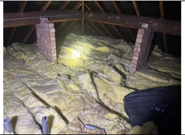
Photo 6 Old dust at loft floor
