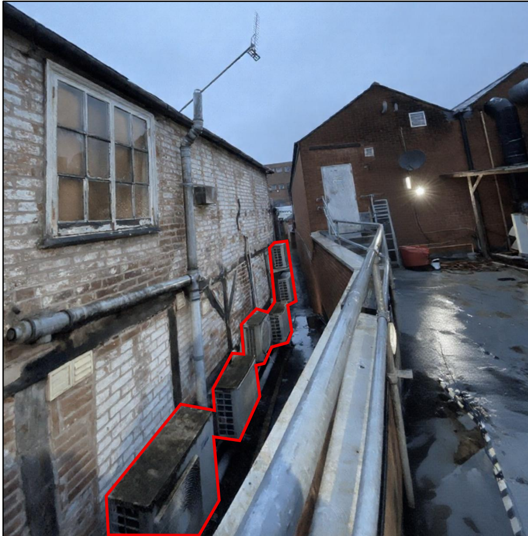
Figure 5: Existing AC units adjacent the first-floor rooftop garden area
