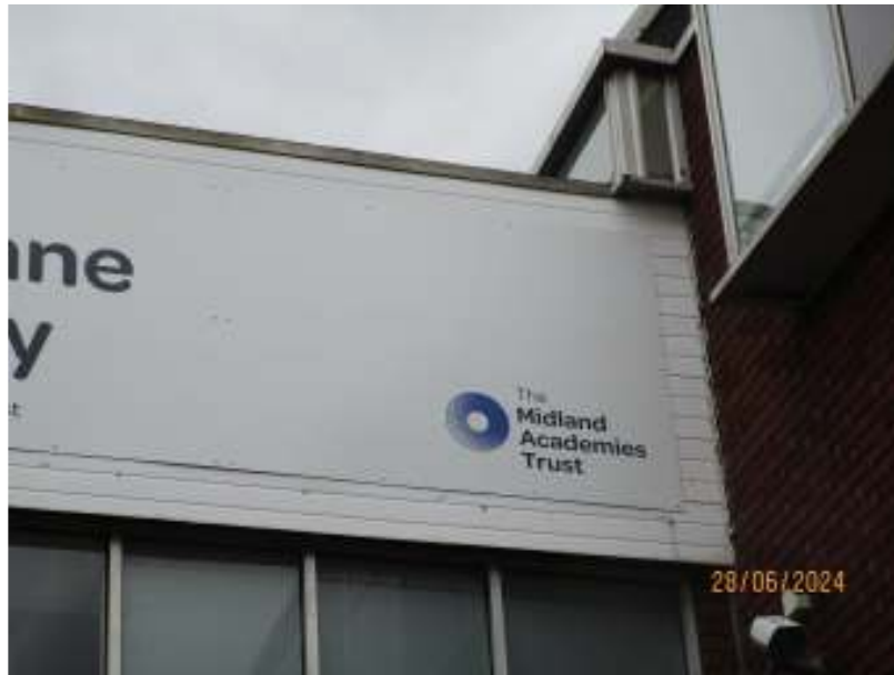
Image 05: Existing white uPVC shiplap cladding damaged by numerous fixing holes to be replaced with new white uPVC shiplap cladding to match the existing. The school signage is to be replaced to reflect the change from 'The Midland Academies Trust' to 'United Learning'.
