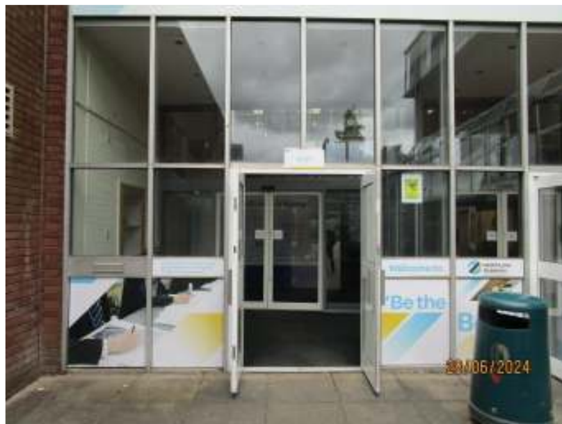
Image 04: Existing manually operated exit doors to be replaced with new fully automatic sliding doors.
