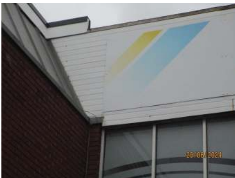
Image 06: Existing white uPVC shiplap cladding damaged by numerous fixing holes to be replaced with new white uPVC shiplap cladding to match the existing. The school signage is to be replaced to reflect the change from 'The Midland Academies Trust' to 'United Learning'.
