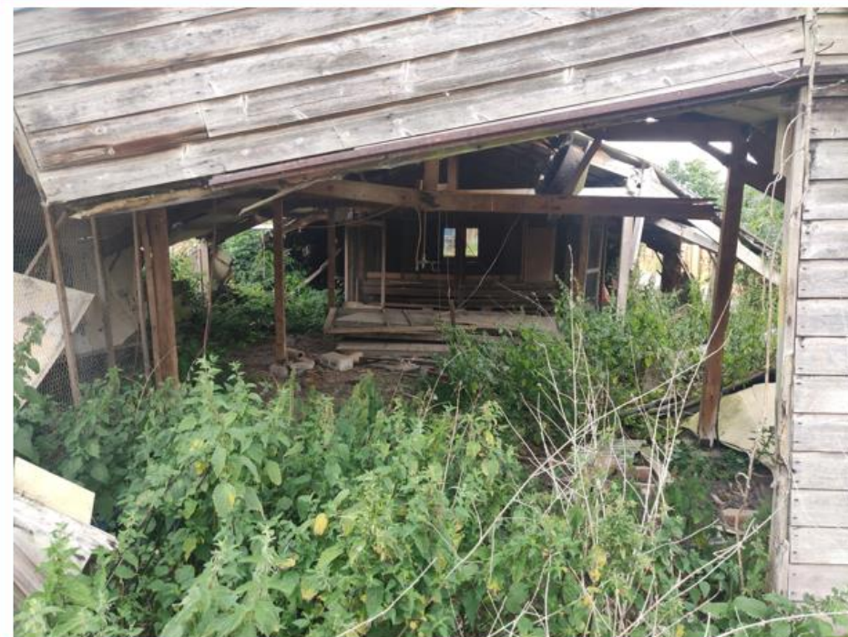
Photo No.16: Facing west from outside the eastern face of the dilapidated linear barn forming the NE extent of site
