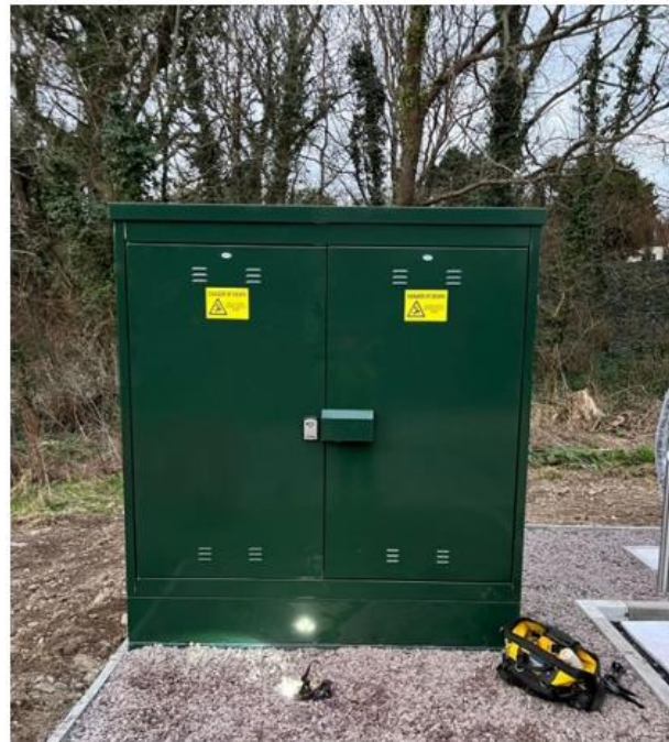
Figure 3: Feeder Pillar RMC 2100
