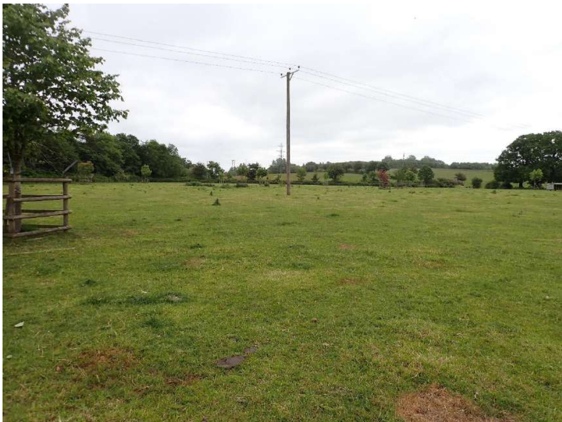
Plate 05: East to West Overhead Service Cable. Field 01.
