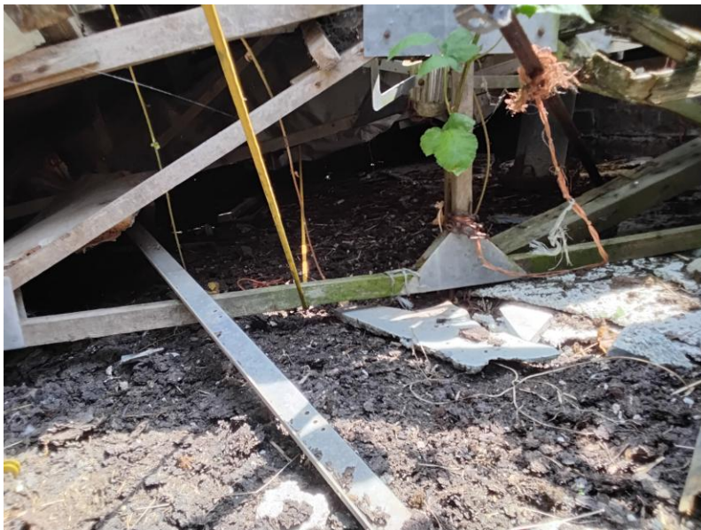
Photos 10 & 11. Lack of digging or sufficient shelter at ID 4 following additional inspection with an endoscope in June 2025
