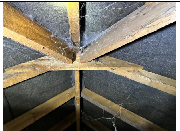
Photo 8 Cobwebbed roof timbers
