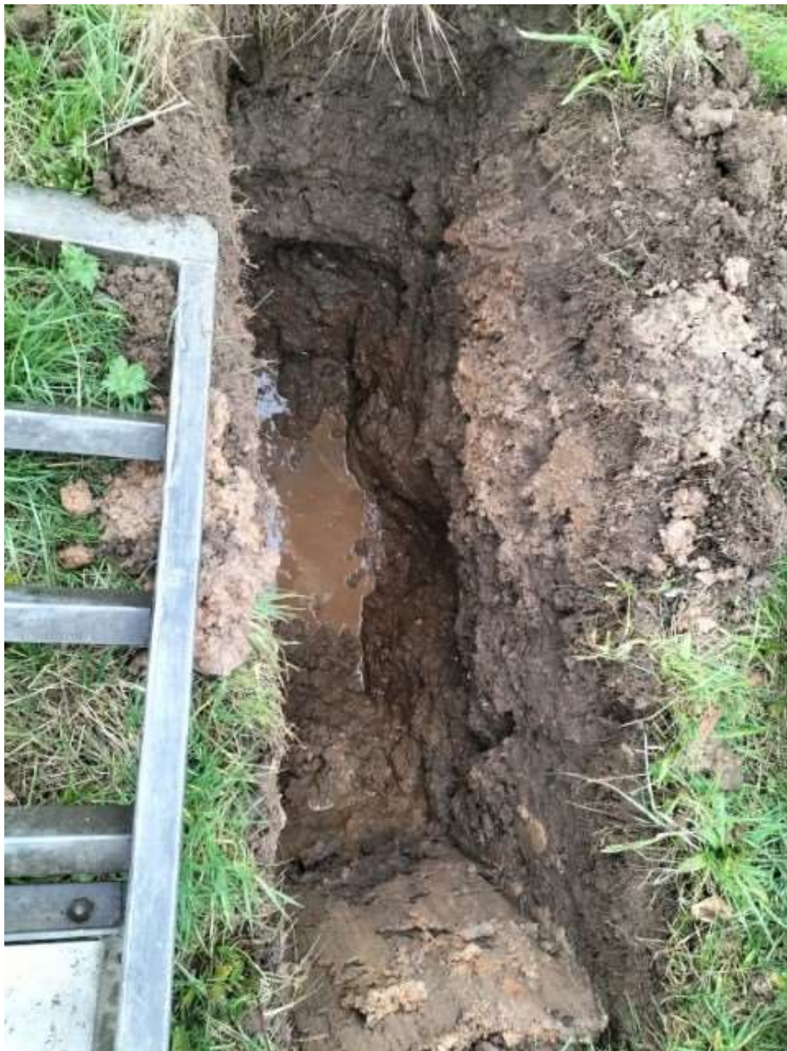
Soakaway test pit TP SA2, showing localised instability due to groundwater ingress.
